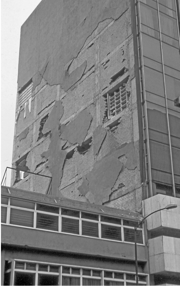
Figure 12.1 Failure of a ‘displacement-sensitive’ non-structural element: façade cladding Mexico City, 1985 (© E Booth)
