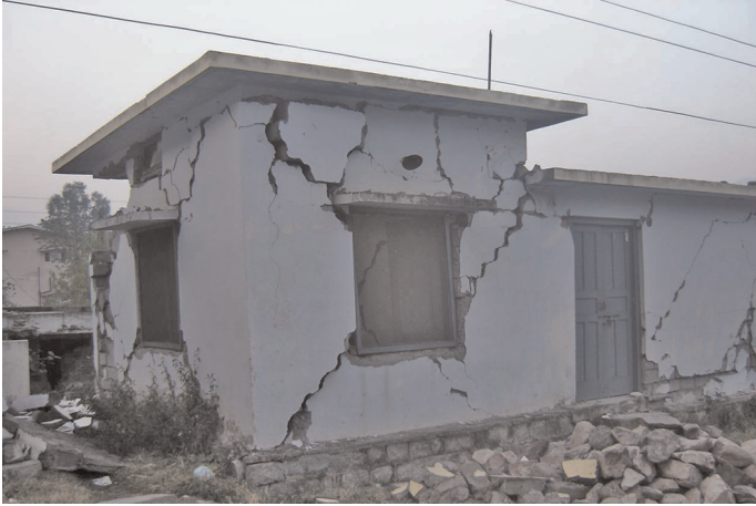
Figure 10.9 In-plane failure of walls in the Kashmir earthquake of 2005 (reproduced from Bothara and Hıçyılmaz, 2008; New Zealand Society for Earthquake Engineering Inc.)
