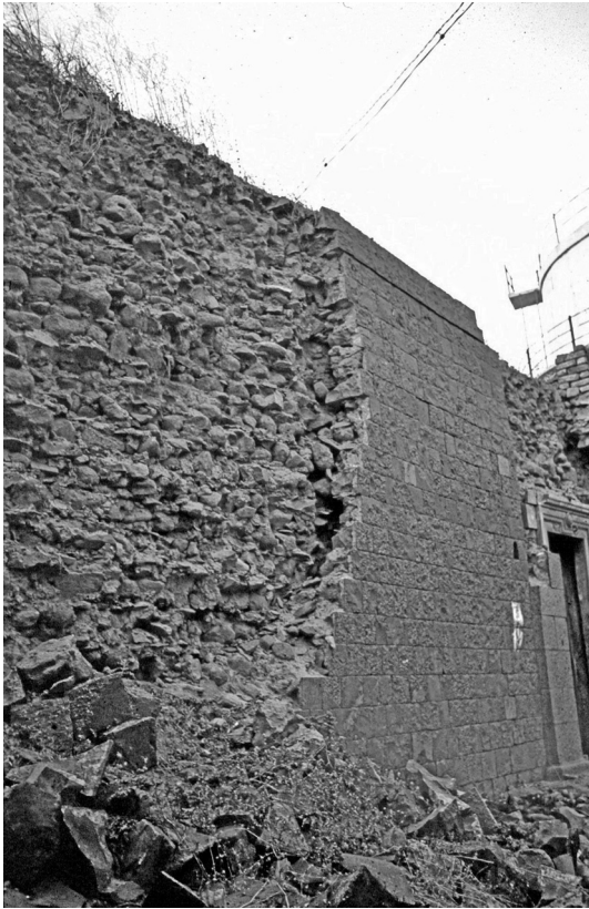
Figure 10.8 Delamination of the outer surface of a wall in the Maharashtra, India earthquake of 1993 (photograph courtesy of S. Brzev)
