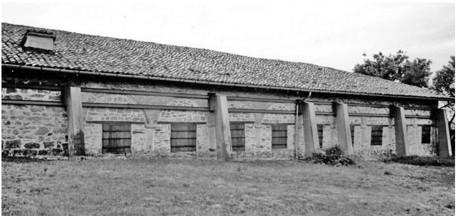
Figure 14.5 Concrete buttresses used to retrofit a historic masonry building in Bulgaria (photograph courtesy of Michael Bussell)
