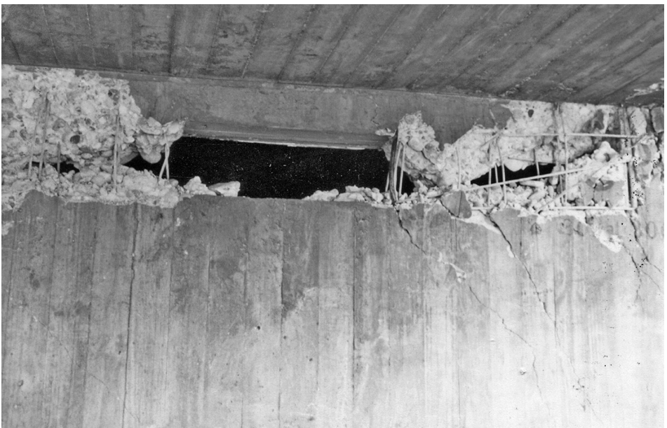
Figure 8.41 Damage around opening in a shear wall, 1985 Chile earthquake (© E Booth)
