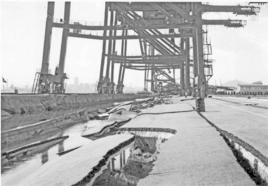
Figure 4.8 Failure of dock wall in the port of Kobe, Japan, 1995
