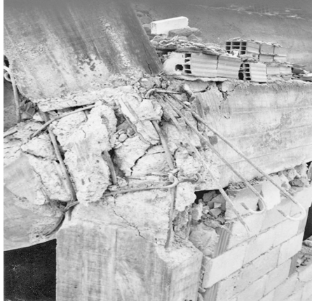
Figure 8.1 Failure of a beam–column joint in Erzincan, Turkey, 1992. Note failure of the concrete in the joint, and bursting out of column steel (© E Booth)
