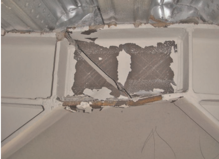
Figure 9.4 Fracture in eccentrically braced frame link in Christchurch, New Zealand, 2011 (reproduced from Clifton et al. (2011); New Zealand Society for Earthquake Engineering Inc.)
