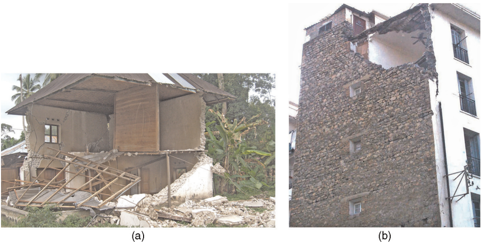
Figure 10.7 Out-of-plane failure of walls: (a) two-storey building, Padang, Indonesia earthquake of 2009; and (b) top floor of six-storey building, Boumerdes, Algeria earthquake of 2003 (a) Reproduced from Bothara et al. , 2010; New Zealand Society for Earthquake Engineering Inc.; (b) photograph courtesy of M. Farsi)
