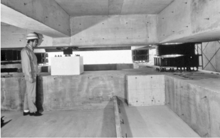
Figure 5.13 Crawl space under a base-isolated building (photograph courtesy of Kajima Corporation, Tokyo)
