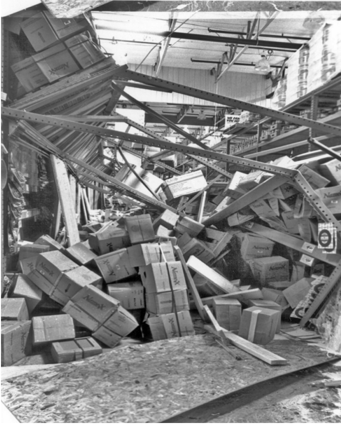
Figure 12.2 Failure of an ‘acceleration-sensitive’ non-structural element: storage racks, Northridge earthquake, California, 1994 (reproduced from BSSC, 2006; image is in the public domain)
