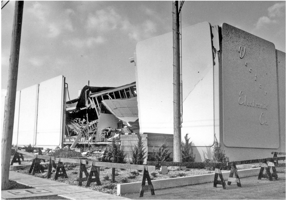
Figure 8.42 Failure of tilt-up warehouse building, Loma Prieta earthquake, California, 1989 (courtesy ABS Consulting, photograph from Peter Yanev, EQE, San Francisco)
