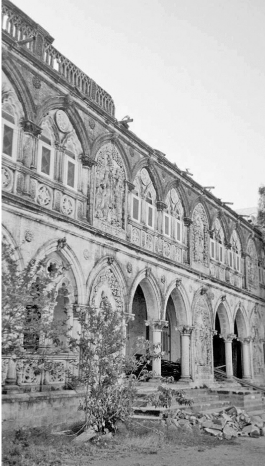
Figure 10.2 Increase in seismic damage with height in a stone masonry building, Gujarat, India, 2001 (© E Booth)
