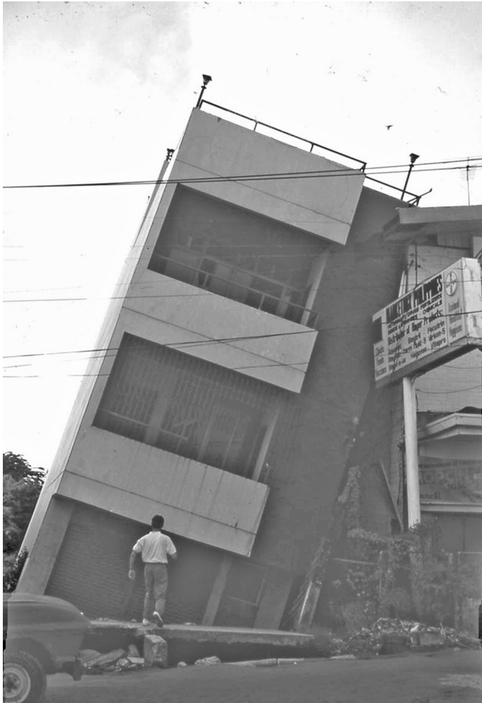
Figure 4.4 Foundation failure due to liquefaction
