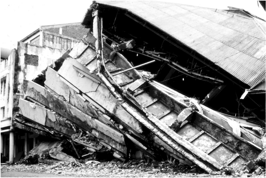
Figure 8.6 Total collapse of a multi-storey reinforced concrete building in Baguio, Philippines, 1990 (© E Booth)
