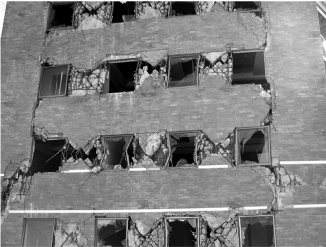
(b) Failure of wall piers, Chile 2010
