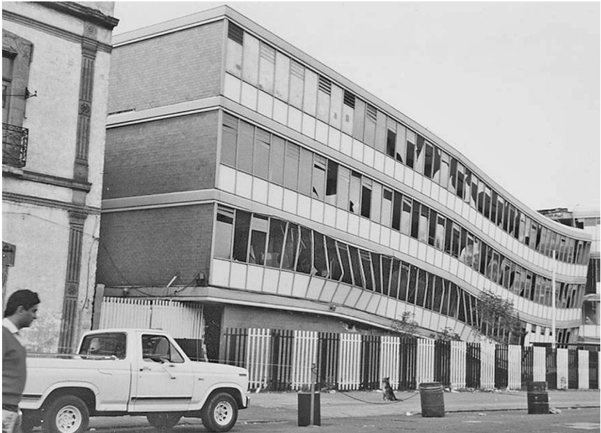
Figure 8.9 The nearer end of this building is restrained by stiff shear walls but the far end was supported by slender columns. The resulting torsional movement has led to collapse in Mexico City, 1985 (© E Booth)
