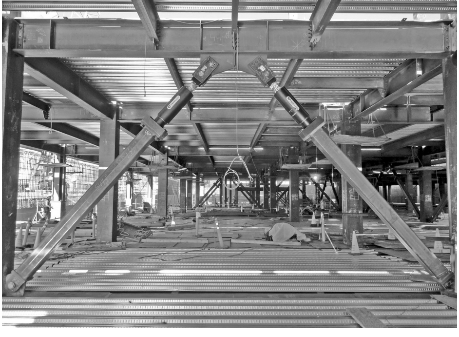
Figure 14.4 Viscous dampers added as retrofit, San Bernardino Justice Center, California, USA (photograph courtesy of Taylor Devices Inc. and SOM (Skidmore Owings & Merrill))
