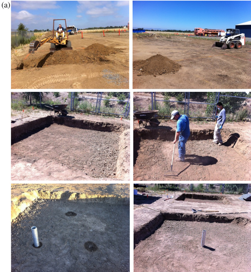
Figure 4.2 Construction of experimental sections for the cool pavement study. (a) Preparation of the subgrade layers. (b) Construction of base layers. (c) Construction of surface layers (paver pavements). (d) Construction of surface layers (concrete pavements). (e) Construction of surface layer (asphalt pavement).
