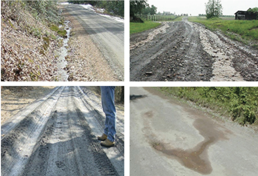
Fig. 1. The damages of the gravel roads (Source: Department of Agriculture, United States)
