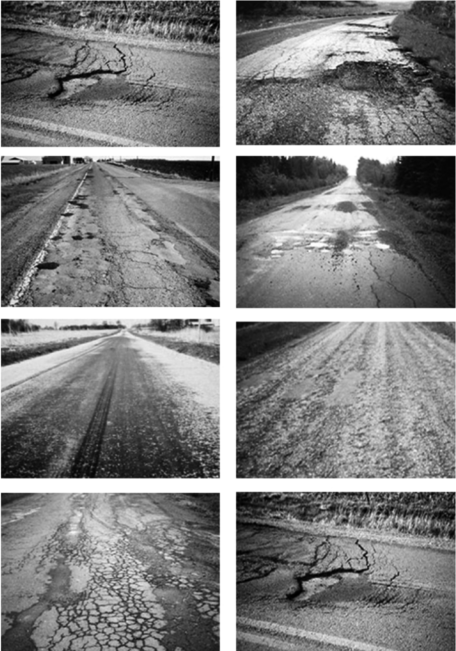
Fig. 2. The damages of the asphalt roads (Source: Walker, 2002)
