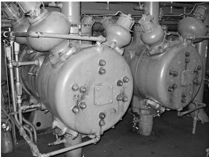
FIGURE 17.3 Three-piece cylinders before revamping. (Source: ACI Services, Inc., Cambridge, OH.)
