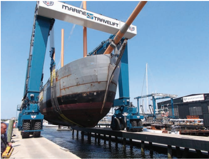
Fig. 10-50. A 500-metric ton capacity Marine Travelift straddle lift installation constructed of cast-in-place concrete runway beams on concrete-filled, rock-anchored steel pipe piles. Note the dual wheel bogies, with four tires per leg
