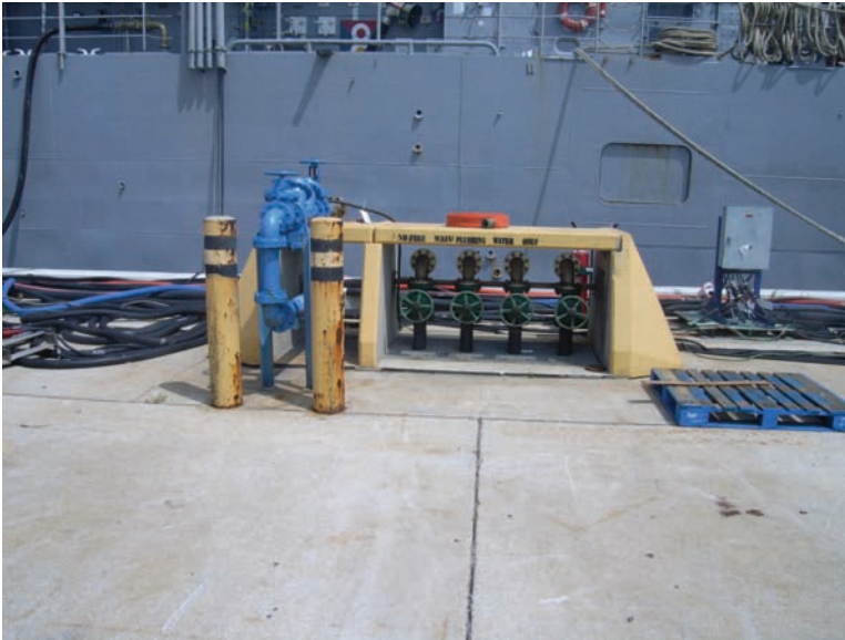
Fig. 7-36. Utility hood protecting risers and valves
