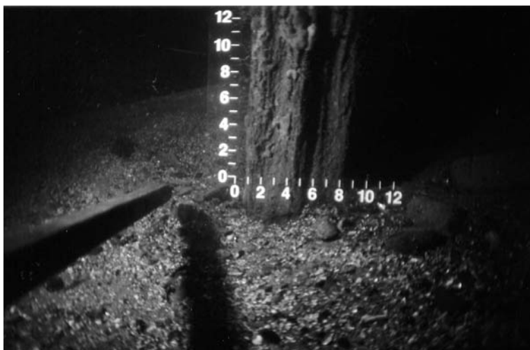
Fig. 11-5. Marine borer damage to wood pile near mudline
