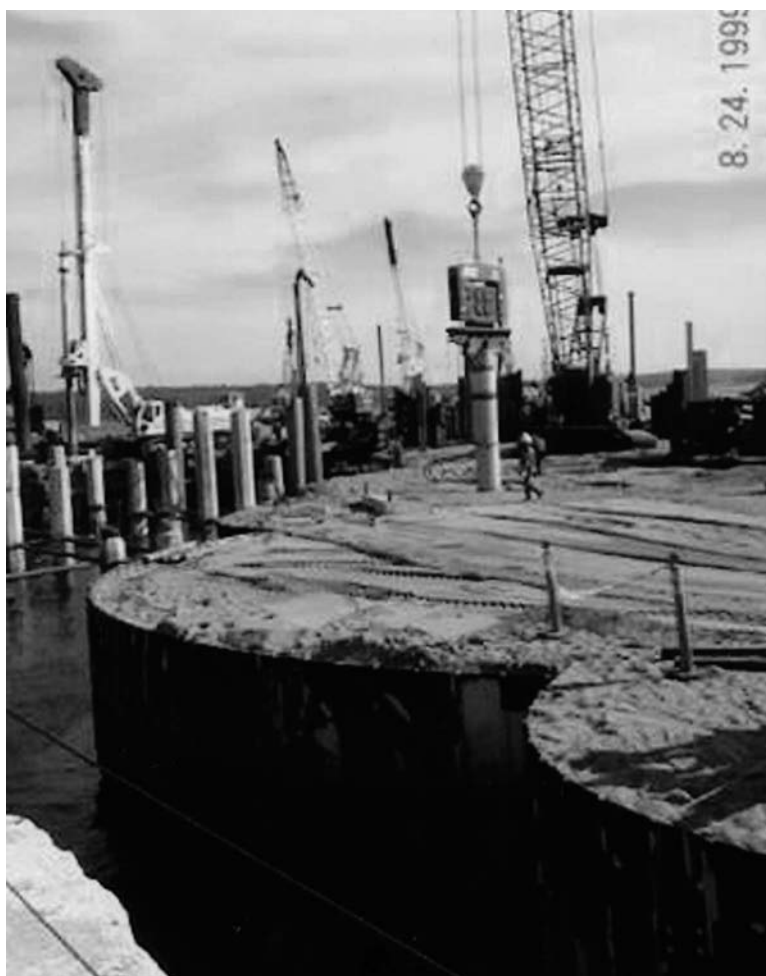
Fig. 8-37. Vibrating probe compaction used to densify loose sand in cofferdam bulkhead to eliminate possible failure caused by earthquake-induced liquefaction
