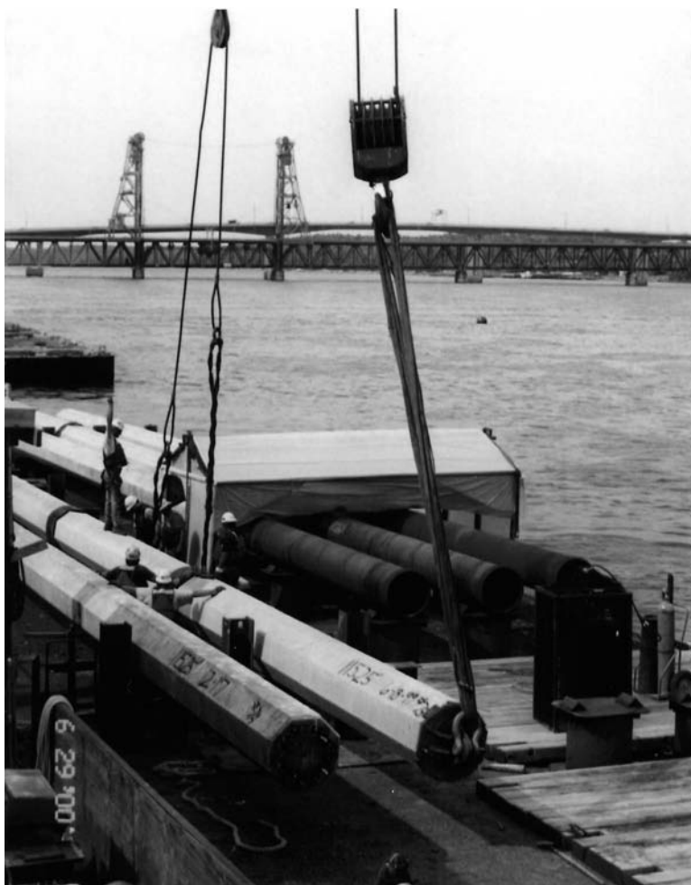
Fig. 8-20. Composite pile consisting of 24-in.-diameter pipe pile welded to a steel plate on the bottom of a 28-in. octagon precast concrete pile
