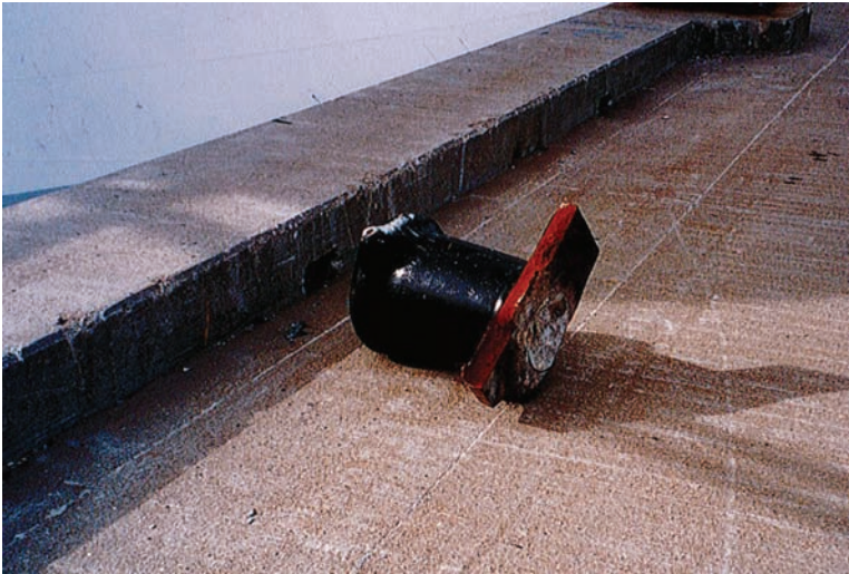
Fig. 11-23. Failed bollard casting caused by initial defect in base that corroded over time, initiating cracking and separation under high mooring line load
