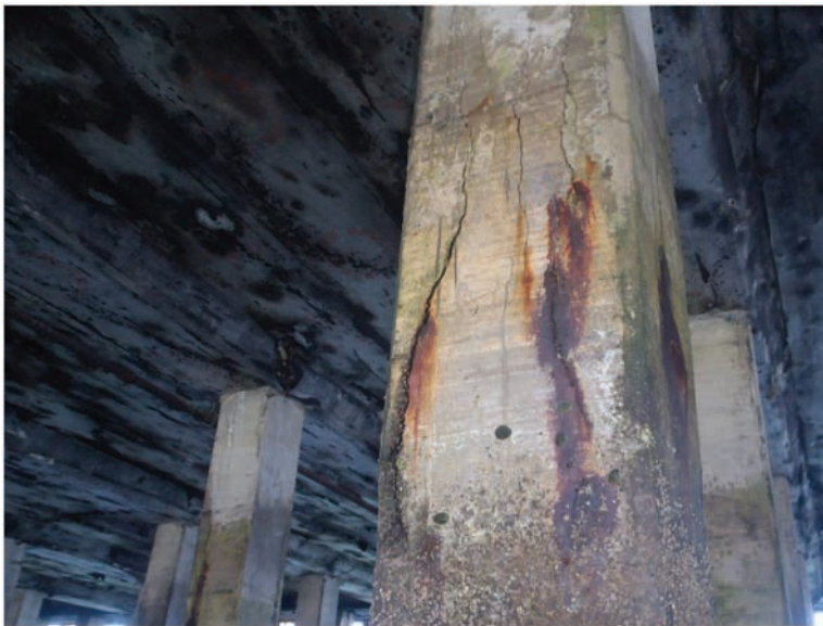
Fig. 12-3. Concrete pile with major cracks and rust staining caused by corroded reinforcing steel
