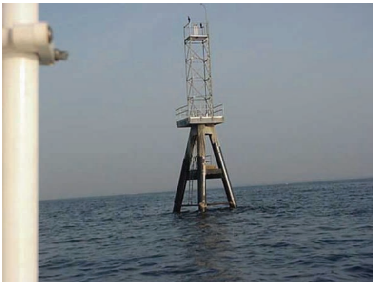
Fig. 7-29. Steel pile tripod ATON structure supporting a range tower with platforms, lights, and solar panels
