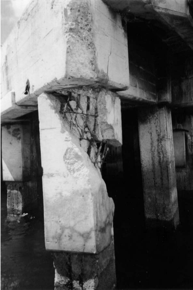
Fig. 11-9. Impact damage to previously repaired concrete pile
