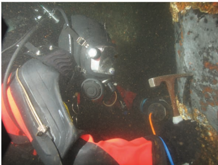
Fig. 12-1. Engineer-diver completing a Level II and Level III inspection of a steel pile
