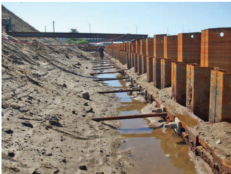
Fig. 11-20. New steel sheet-pile bulkhead driven outside of existing deteriorated bulkhead and using existing tieback anchor rods with new anchor bolts securing new internal wale system to existing wale on opposite sides of sheeting
