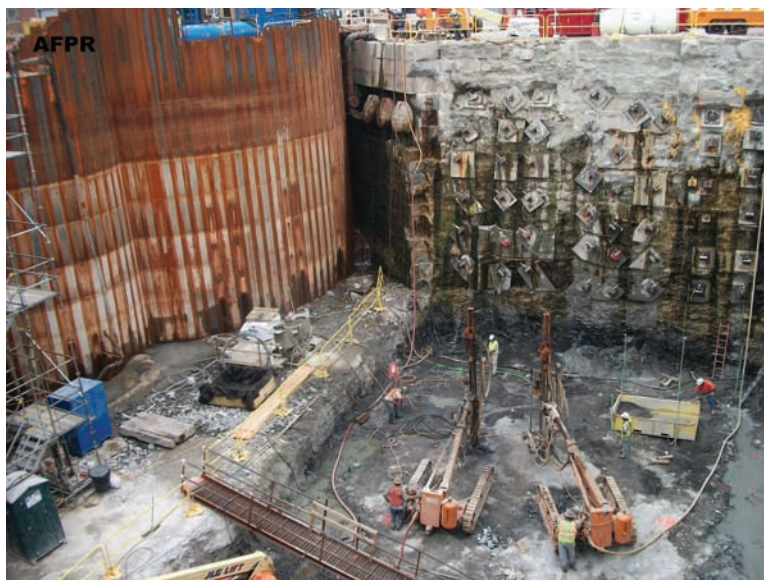
Fig. 11-13. Major rehabilitation of basin dry dock floor and walls involving extensive removal of concrete and granite block facing and installation of prestressed rock anchors to anchor floor and walls against hydrostatic pressures. Note sheet pile cells for temporary end closure
