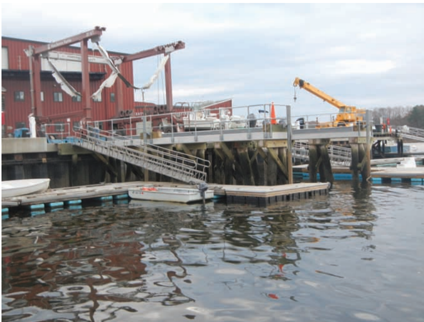
Fig. 10-49. A 35-metric ton capacity boatyard straddle lift installation constructed of precast concrete runway beams on a braced greenheart timber pile foundation
