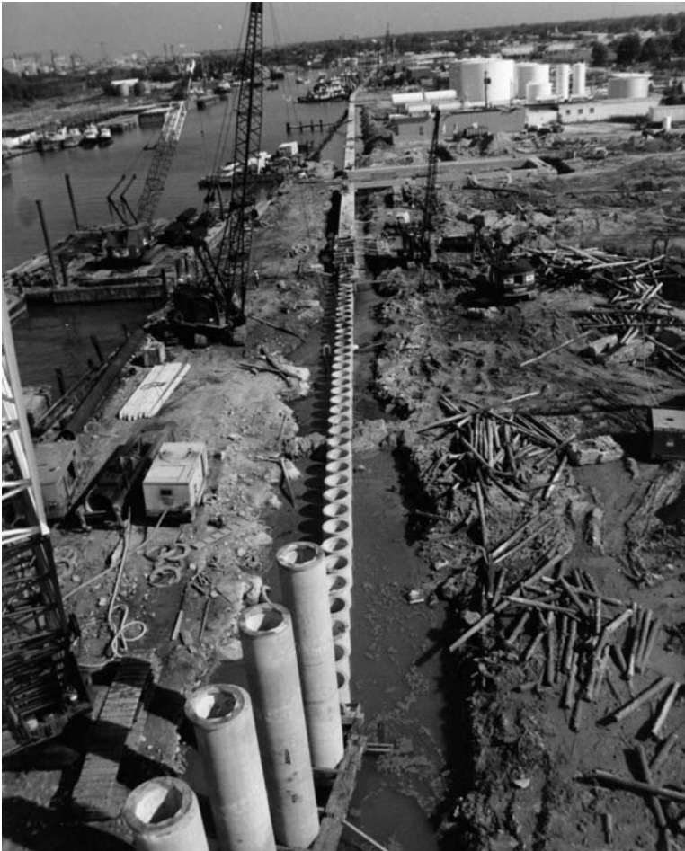
Fig. 8-9. Prestressed concrete cylinder piles used as a cantilevered retaining wall, City of Newport News, Virginia, Seafood Industrial Park
