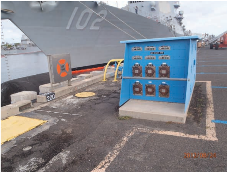
Fig. 7-37. Electrical services vault
