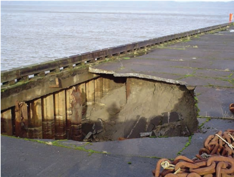
Fig. 11-11. Failed pavement and washout of fill behind steel sheet pile bulkhead caused by loss of fill through severely corroded bulkhead
