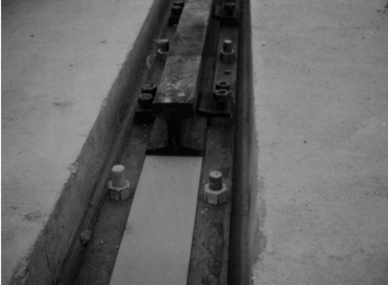
Fig. 7-31. Installation of crane rail for shipyard gantry crane before grouting below rail plate. Note anchor bolts, rail clips, and bearing pad
