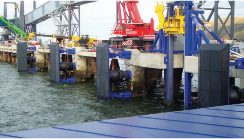
Fig. 5-18. Parallel motion-type fenders with back-to-back mounted cones at an open pier structure supporting a conveyor system
