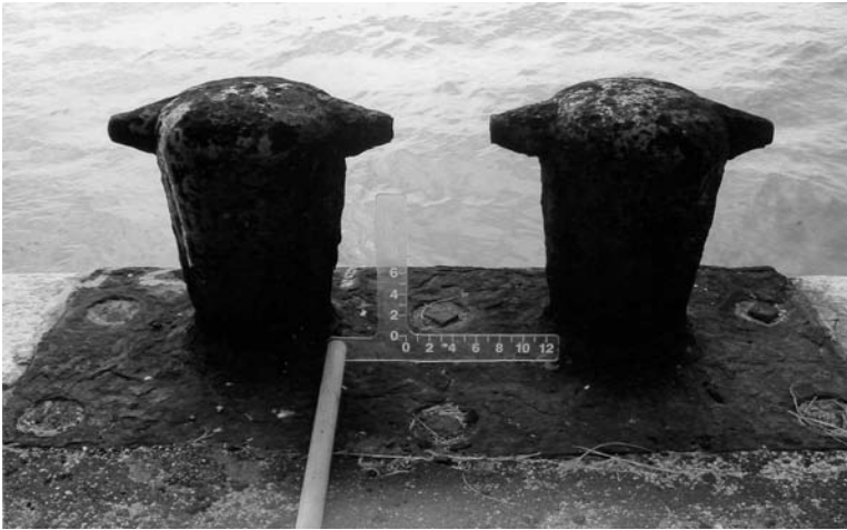
Fig. 11-1. Severe corrosion of a double bitt
