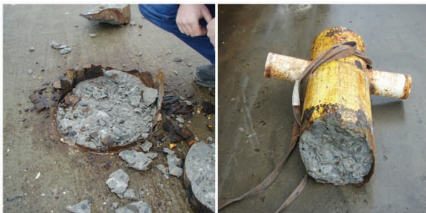
Fig. 12-6. Steel pipe bollard that failed because of section loss within high corrosion zone
