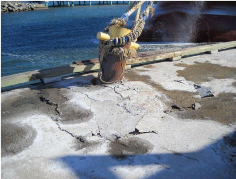
Fig. 11-10. Failed concrete deck because of bollard pullout likely caused by poor design of deck and anchorage and deterioration of concrete combined with high mooring line load
