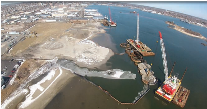
Fig. 8-15. Circular steel-sheet-pile cofferdam bulkhead, showing construction sequence, New Bedford, Massachusetts, Marine Commerce Terminal
