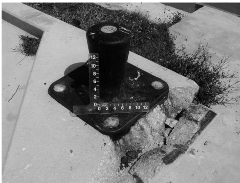
Fig. 11-22. Typical concrete pedestal damaged by corrosion expansion of embedded cast-steel bollard
