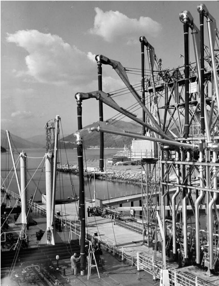
Fig. 4-9. Hose loading tower with 8- and 12-in. flow booms at Finnart Refinery in Scotland
