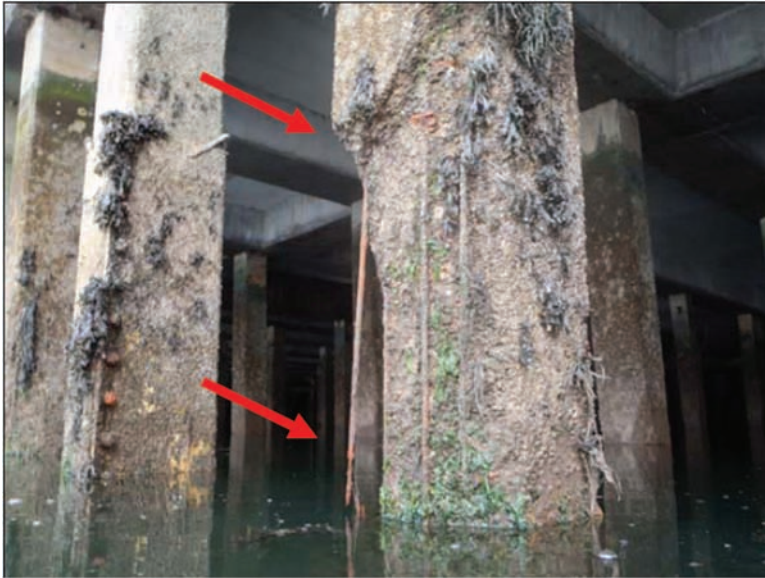
Fig. 12-9. Severely deteriorated concrete pile; note exposed and corroded steel reinforcement
