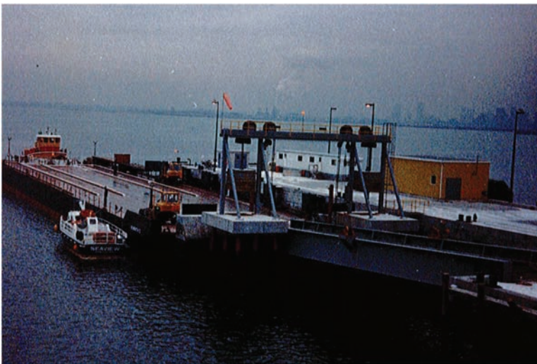
Fig. 9-15. Transfer bridge with fixed adjusting tower for offloading of construction equipment and supplies from barges. Note wire rope reeving and counterweight system for operating bridge
