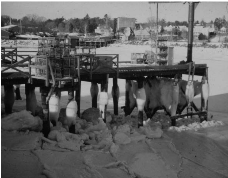
Fig. 4-15. Light-timber pier encumbered with ice. Note coverage of cross bracing and ice collars on piles
