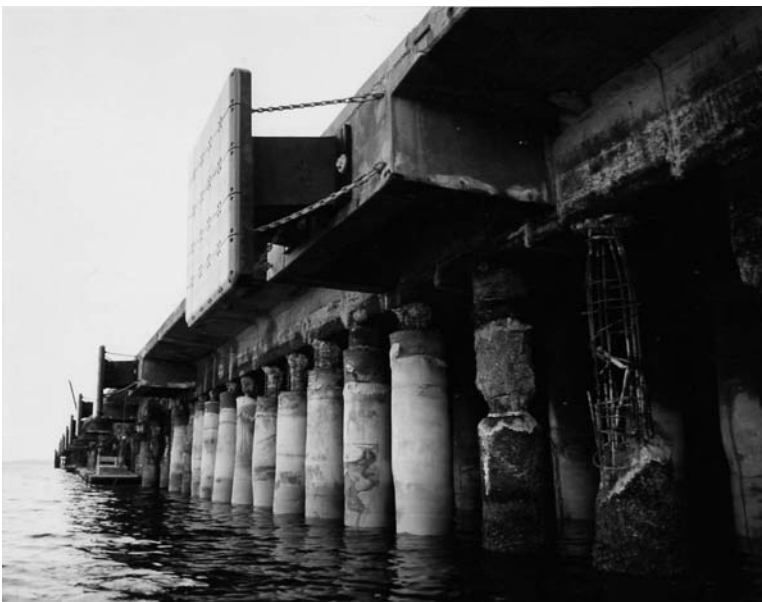
Fig. 11-8. Deterioration of concrete pile shafts in the tidal zone. Piles to the left have been partially restored by the use of concrete-filled fabric forms. Installation of contemporary resilient fender units helps reduce berthing impact loads
