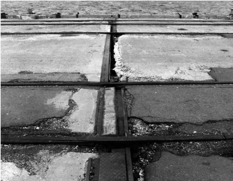
Fig. 11-7. Degradation of concrete wharf deck at expansion joint and rail pockets. Bituminous patches have likely accelerated the deterioration
