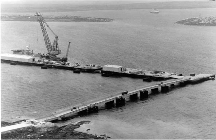
Fig. 9-2. Falkland Islands “Flexiport” under construction. Access bridge is supported on removable submerged pontoons
