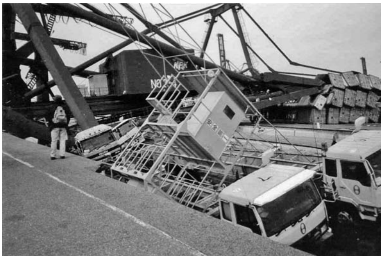
Fig. 4-19. Earthquake liquefaction damage to container terminal wharf, Rokko Island, Kobe Port, Japan, January 1995
