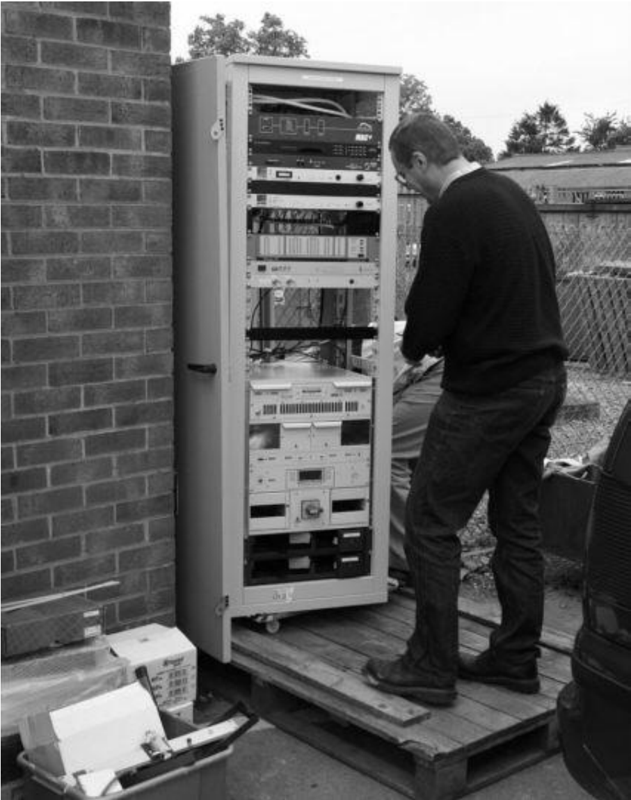
Tim Foulsham of transmission supplier Radica installs a pre-wired rack including all the equipment needed for transmission and back-up studio links for a local FM service. Photo: Brian Lister
