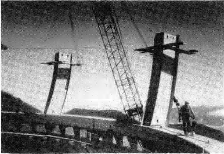
Steel girders going in place on the Keck I dome. (Courtesy Keck Observatory)
