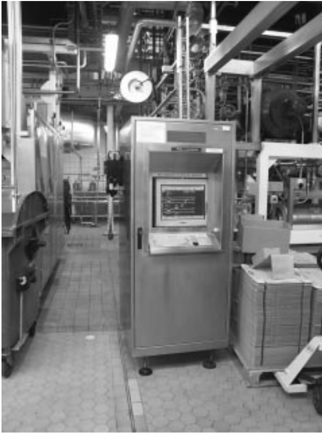
Fig. 15.4 Stainless steel cabinet placed 100 mm from the floor.
