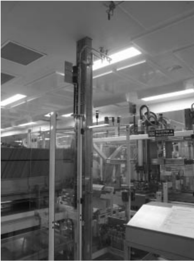
Fig. 15.5 Walkable ceiling with integrated luminaires above the conditioned production zone H and a vertical cable trunk to the machine.
