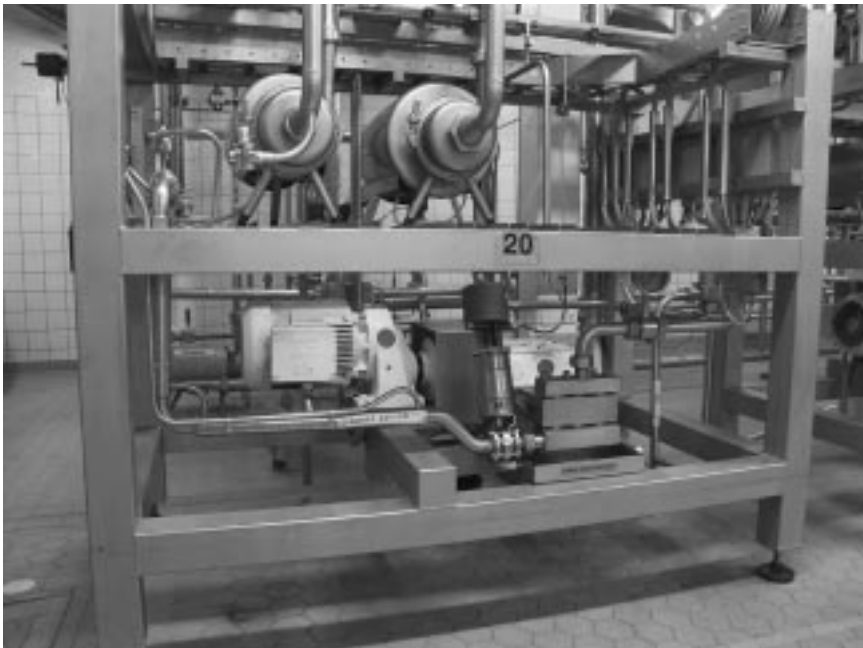
Fig. 15.2 Well cleanable and maintainable setup of equipment in Zone M.
