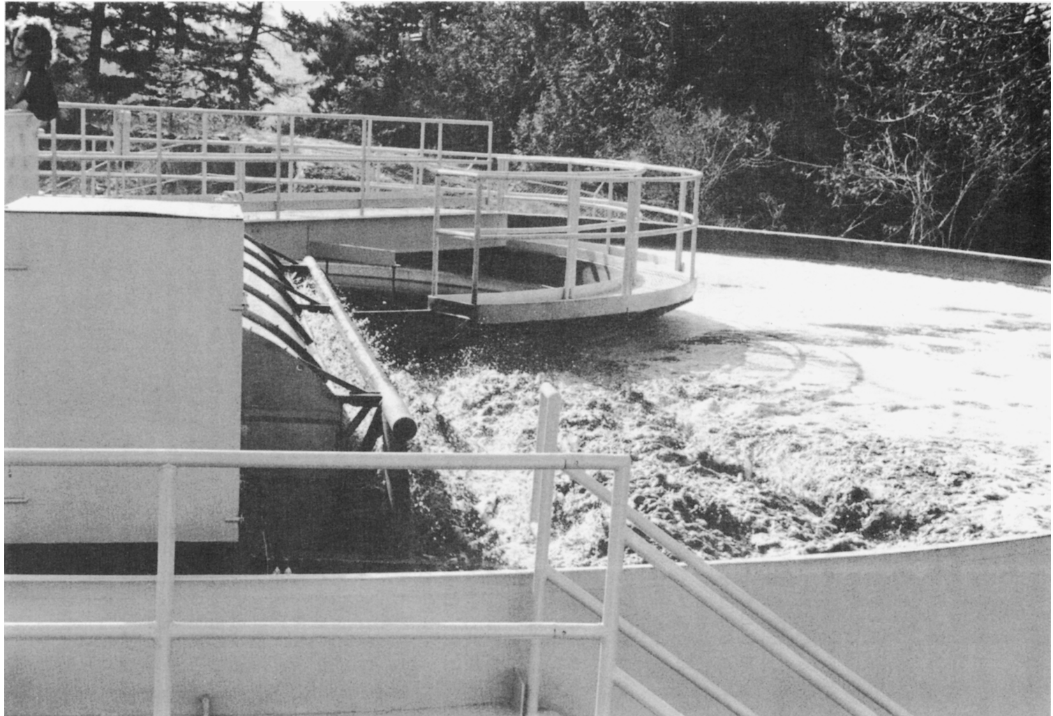
Activated sludge aeration stage for a smallscale secondary sewage treatment plant operating at Central Saanich, British, Columbia.
