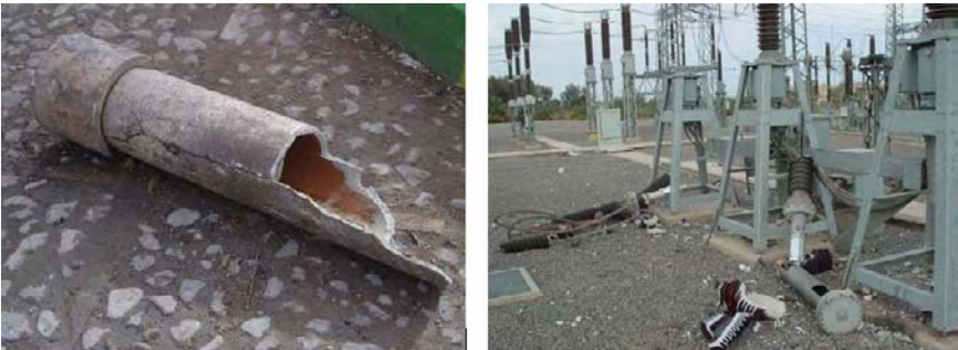
Figure 1: Damaged Bam asbestos cement water pipe and electric substation.
