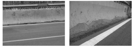
(a) Reinforced concrete crash barrier walls on the Songhua River Highway Bridges (1986)
