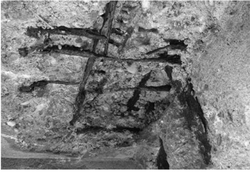
Figure 2. Heavy corrosion was affecting rebars, sometimes up to complete loss of section.
