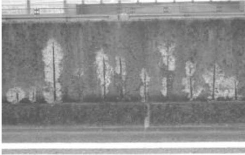
Figure 2. Deteriorated RC wall in bridge.
