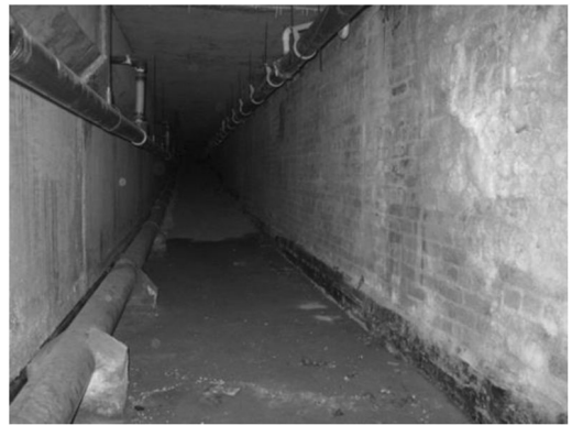
Figure 4. Evidence of standing water in dry duct due to expansion joint leakage.
