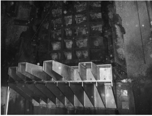
Figure 8. Installed stainless steel toothed plate weir as replacement for original trough structure.
