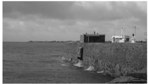
Figure 14. Water flowing out of masonry after wave passes.
