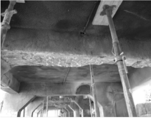
Figure 12. Removal of loose cover, repair and protection of concrete during full access survey and repairs.
