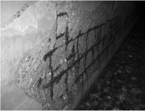
Figure 8. Delamination and corrosion at wet duct wall.
