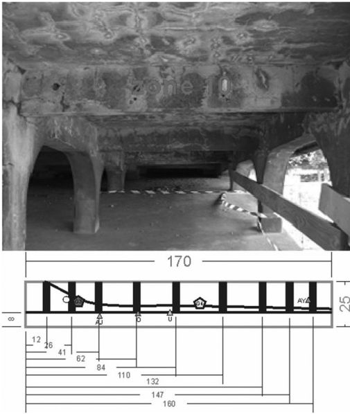
Figure 8. Atypical rebar network electromagnetically detected on zone 10, mixing 2 standard round shaped-rebars (one horizontal and one oblique, both 20 mm in diameter) and 9 flat Hennebique stirrups (4 to 4.5 cm large). On the scheme: the two pentagonal-shaped points refer to the Rp measurement spots, the white dot corresponding to the connecting point. The four triangular-shaped points refer to the powders drilled respectively before treatment (O), just after treatment (U), 2 months after (AJ) and one year after (AY).
