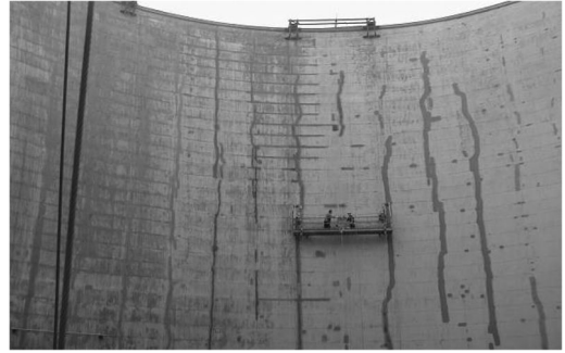
Figure 10. Deep cracks covered over by special coating.
