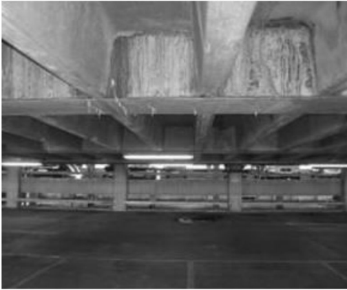
Figure 1. General condition of the MSCP's soffit indicating leaching, dynamic cracking and deterioration of the concrete elements.
