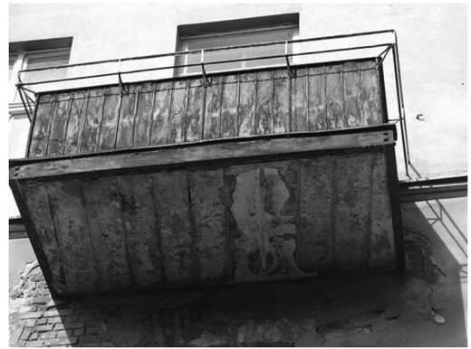
Figure 14. Concrete destruction in “Stolte” slab.
