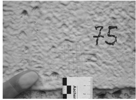
Figure 3. Chalking surface of epoxy coating due to photo-catalytic degradation process.
