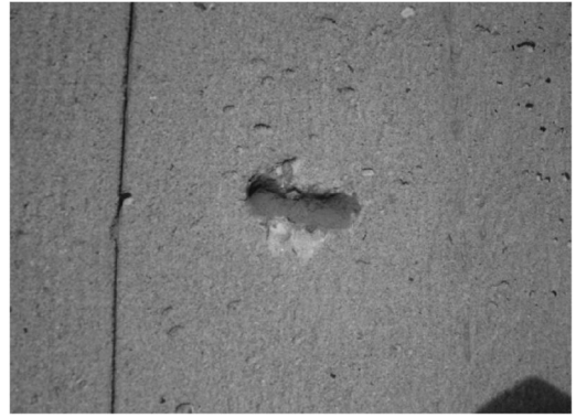
Figure 5. Example of previous repair using proprietary system.
