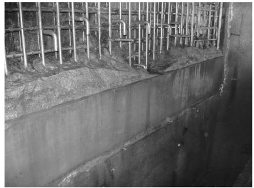
Figure 7. Bypass wall under the penstock strengthened using grade 316 stainless steel bars and dry spray (lower section) and flowable (upper section) calcium aluminate concrete, location of the pour break after pump malfunction.
