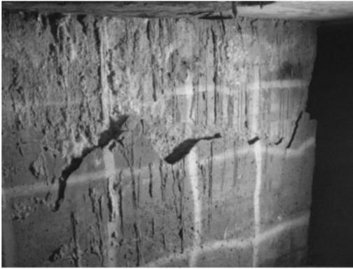
Figure 5. Delamination of pool wall in dry duct.
