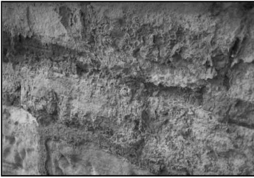
Figure 5. Poor condition, deteriorated stonework (S).
