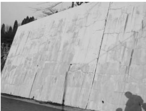
Figure 1. Example of re-deteriorated repair system.
