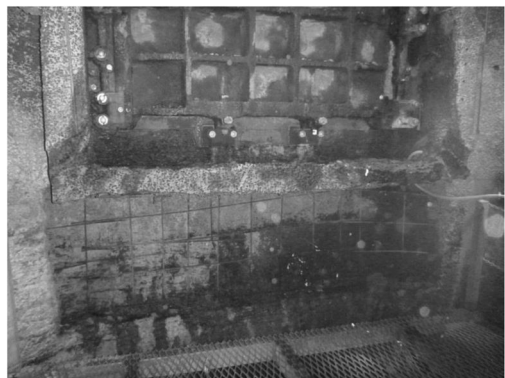
Figure 1. Bypass wall under penstock gate after hydro-demolition of acid damaged concrete and prior to initial remedial work.
