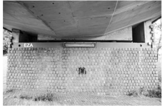
Figure 8. EZA installed on the beams supporting the bearings of the Hubertus viaduct in The Hague.
