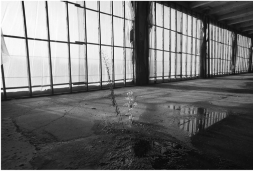
Figure 3. New York Dock Building Today. Note thin polystyrene sheets as weatherproofing and standing water and the formation of plant growth at saturated slab. Author's photograph.
