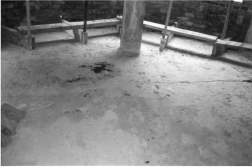
Figure 3. Large crack on the overhanging slab in the first floor.
