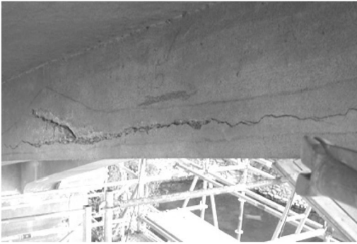
Figure 3. Some of the beams were deeply cracked.
