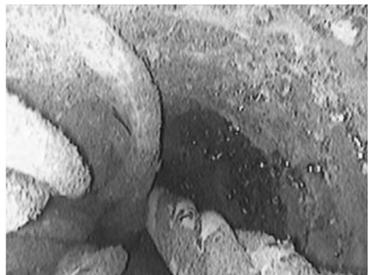
Figure 5. Failed strands in ungrouted duct.
