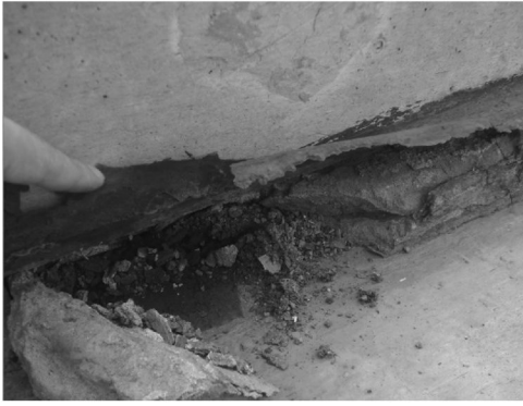
Figure 1. Damage of emulsified asphalt cement mortar layer.
