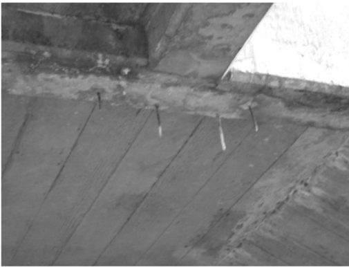
Figure 4. Stalactites forming due to water leakage.
