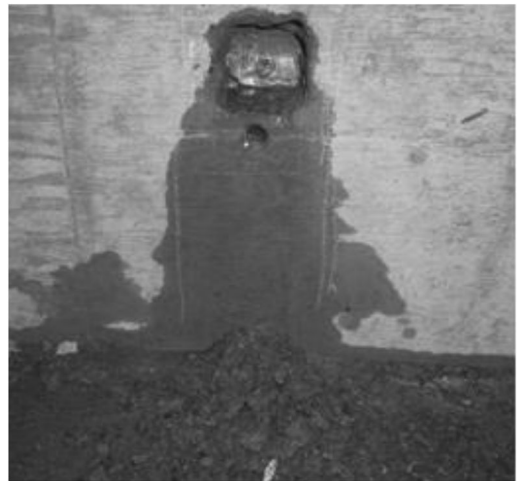
Figure 4. Voided duct containing water.
