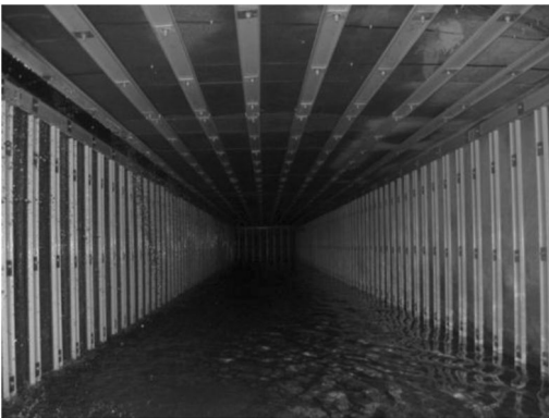
Figure 9. Installed cassette system.
