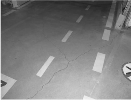
Figure 2. Cracks in an industrial floor.
