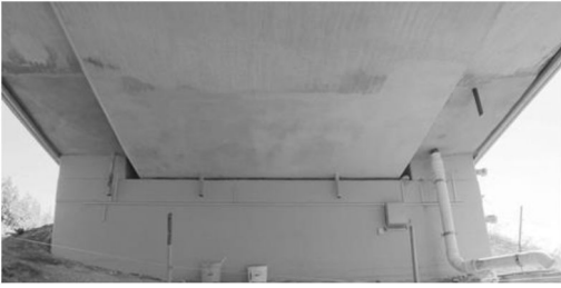
Figure 3. View on the EZA installed on the abutment of the Aplgrabenbridge.
