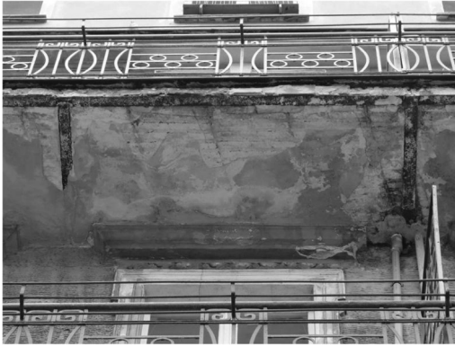
Figure 12. Destruction of “Wygasch” slab.
