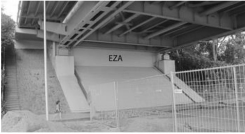
Figure 6. De Meerenbrug steel bridge with EZA installed on the concrete abutment.
