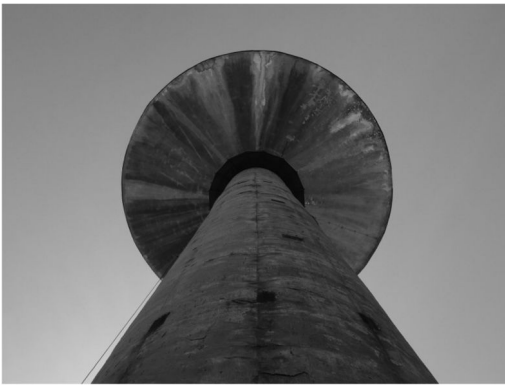
Figure 4. View of the shaft with cracks, cover cavities and exposed corroded reinforcement.
