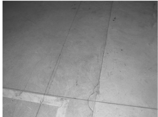
Figure 1. Cracks in an industrial floor.
