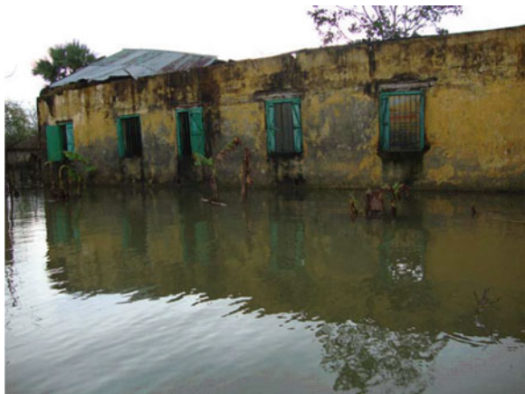
Fig. 15.9 Fully damaged school [ Source Jagrata Juba Shanga (JJS 2009)]
