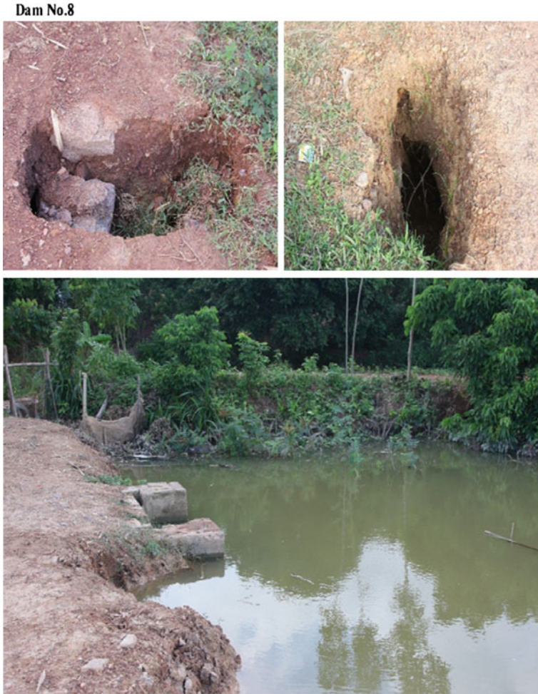
Fig. 29.6 Piping failure resulting from construction or material defects and inappropriately designed spillway
