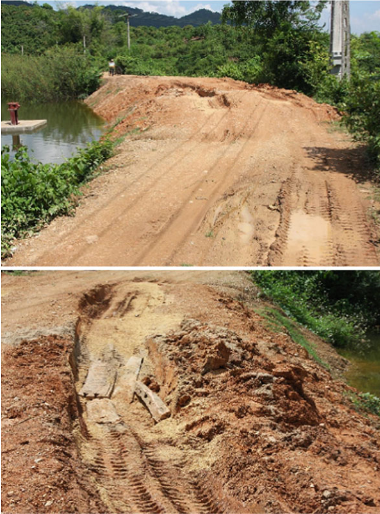
Fig. 29.4 Severe traffic damage on the crest
