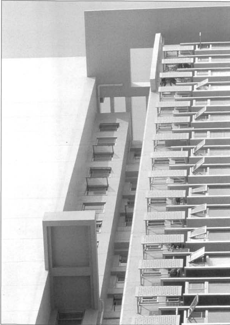
Plate 2 Cantilevered roof: Extended roof surface area for solar collection while providing supplementary solar-shading and insulation.
