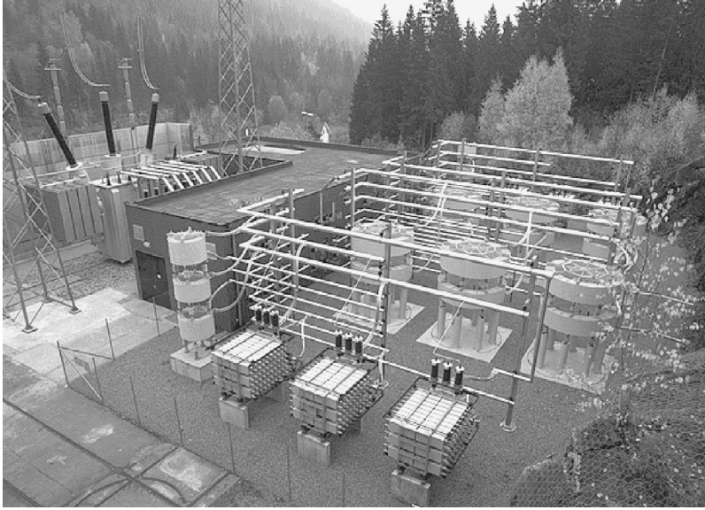
FIGURE 18.1 View of static VAR compensator (SVC) installation. (Photo courtesy of ABB.)
