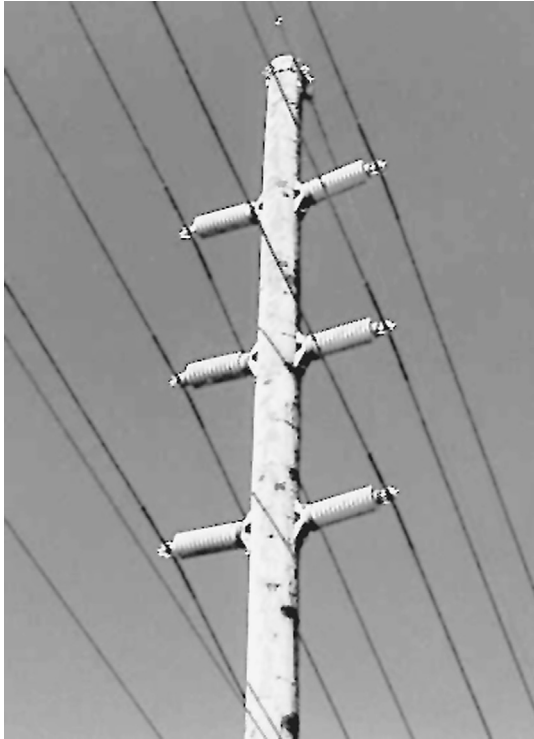
FIGURE 10.2 69-kV transmission line with post insulators.
