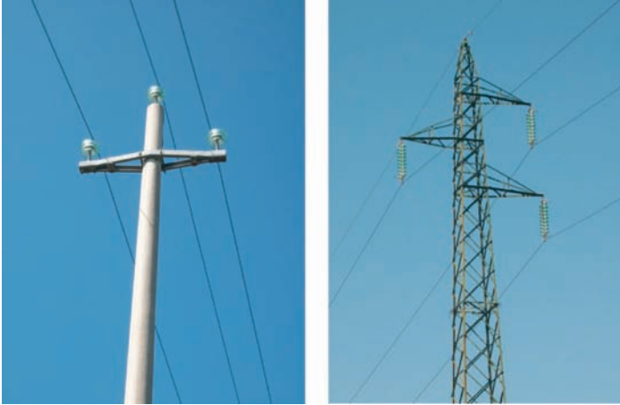
FIGURE 6.1. Two three-phase overhead lines ( left: medium voltage; right: high voltage ).
