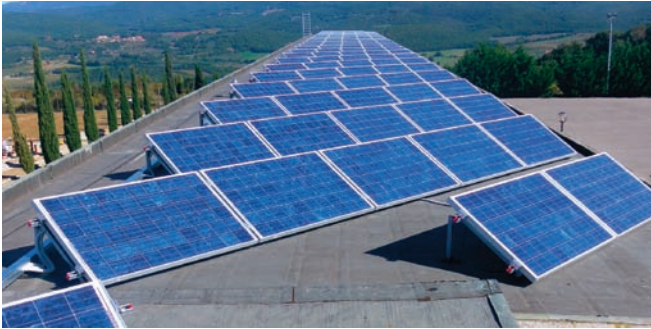
FIGURE 15.18. Photovoltaic panels installed on a roof.
