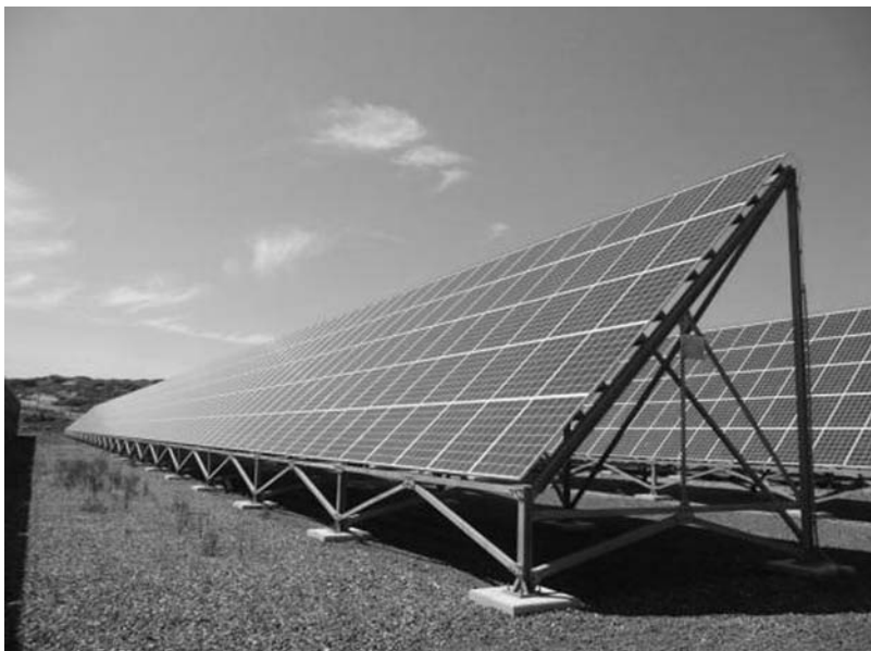
Figure 8.36 Solar array of a large-scale photovoltaic power plant [30]
