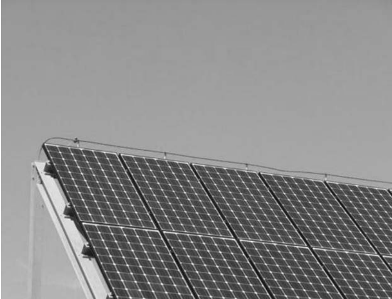
Figure 8.37 Lightning conductor on a structure of a solar array [30]
