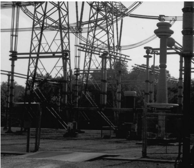
FIGURE 6.11 An 800 kV disconnect switch on the ac side at the same converter station.
