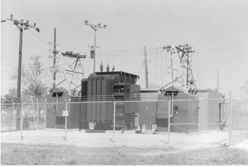
FIGURE 2.39 A distribution substation operating at 34.5/4.16 kV voltage level. (Union Electric Company.)
