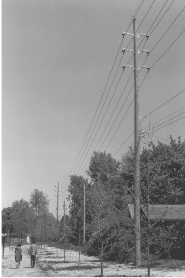
FIGURE 2.32 A typical 34.5 kV line with a double circuit and wood poles. It has a newer style construction. (Union Electric Company.)
