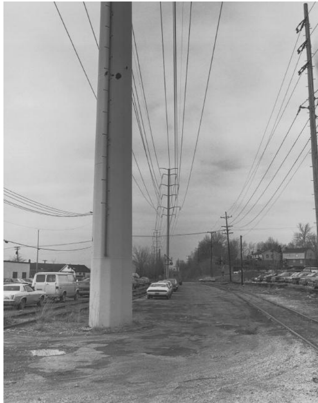
FIGURE 2.6 A double-circuit 138 kV line built by using steel poles, having two 138 kV circuits underbuilt. (Union Electric Company.)
