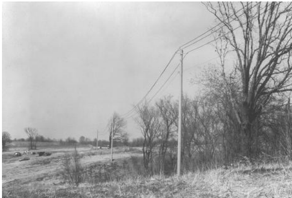
FIGURE 2.35 A typical 12.47 kV line with a single circuit and wood pole. It has a newer type of pole-top construction. (Union Electric Company.)
