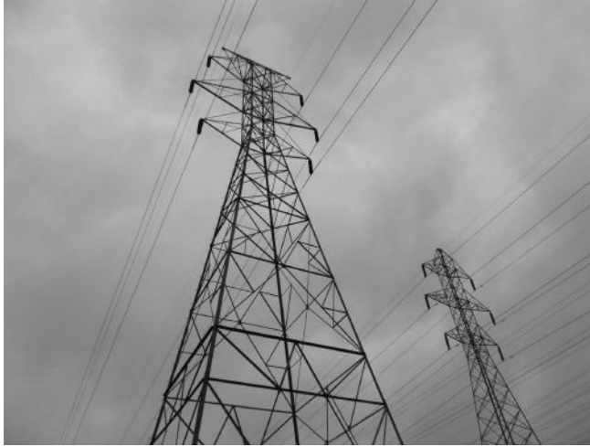
FIGURE 2.22 A 345 kV transmission line and a 115 kV transmission line side by side. (Courtesy of West Power Inc.)
