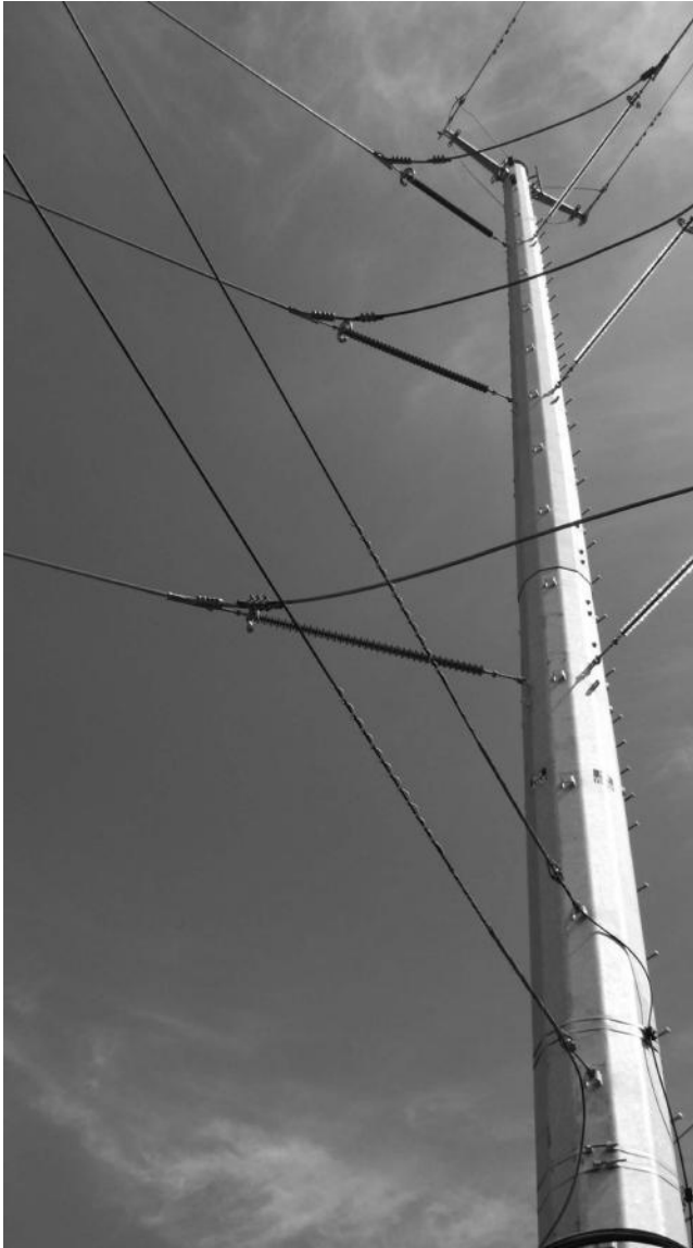
FIGURE 2.26 A galvanized dead-end corner pole of a 230 kV transmission line. (Courtesy of West Power Inc.)
