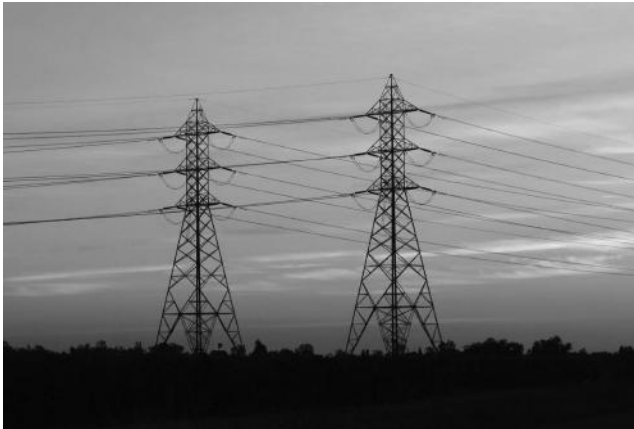
FIGURE 1.1 A three-phase double-circuit transmission line made of steel towers.
