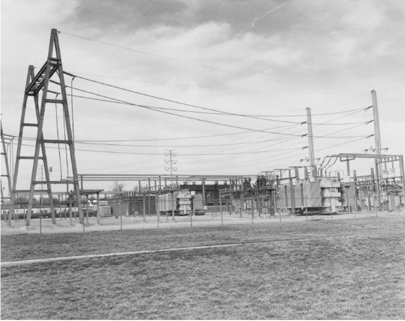
FIGURE 2.37 A bulk power substation operating at 138/34.5 kV voltage level. (Union Electric Company.)
