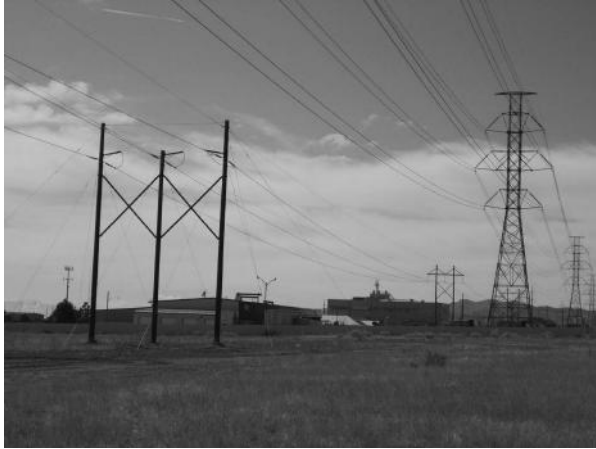
FIGURE 2.19 A 115 kV transmission line and a 230 kV transmission line side by side. (Courtesy of West Power Inc.)
