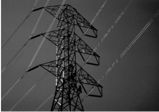
FIGURE 2.14 A typical 230 kV transmission line steel tower with bundled conductors and double circuit.
