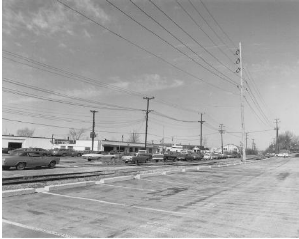
FIGURE 2.34 A typical 34.5 kV line with a double circuit and wood poles. It also has a 4.16 kV underbuilt line and a 34.5 kV switch. (Union Electric Company.)
