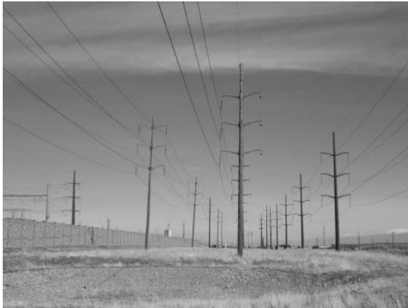
FIGURE 2.20 A cluster of four transmission lines side by side. (Courtesy of West Power Inc.)
