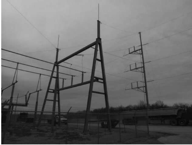
FIGURE 2.27 A substation connection of transmission lines. (Courtesy of West Power Inc.)
