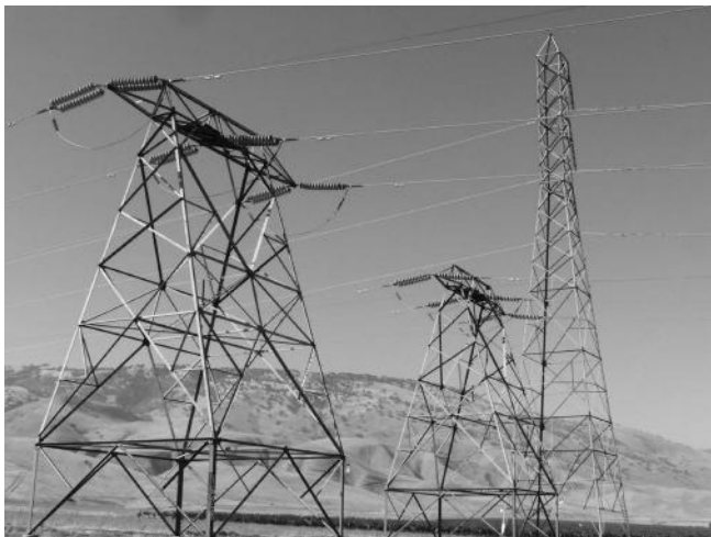
FIGURE 2.16 Two 345 and 230 kV transmission lines side by side. (Courtesy of West Power Inc.)
