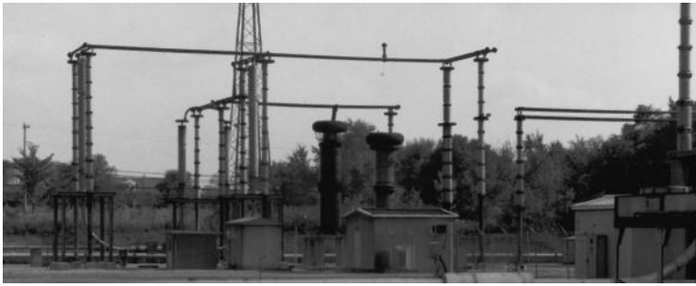
FIGURE 6.10 800 kV dc terminals of a converter station.
