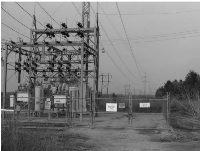
FIGURE 2.18 A 230/161 kV substation with a 230 kV transmission line passing by. (Courtesy of West Power Inc.)
