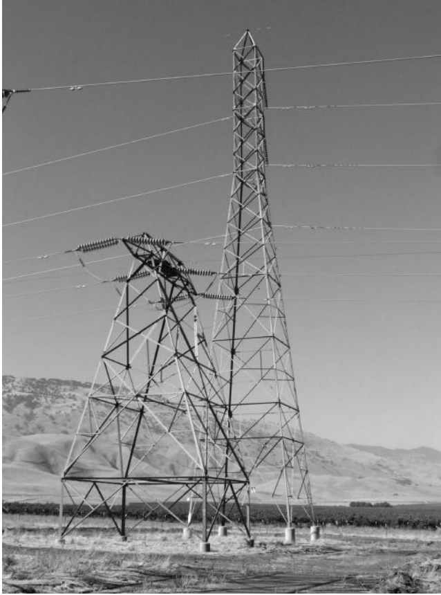
FIGURE 2.17 A 345 kV transmission line and a 230 kV transmission line side by side. (Courtesy of West Power Inc.)
