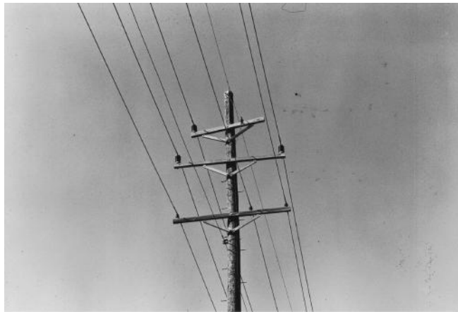
FIGURE 2.33 A 34.5 kV line with a single circuit and wood poles. It also has a 12.47 kV underbuilt line and 34.5 kV switch. It has an old style construction. (Union Electric Company.)
