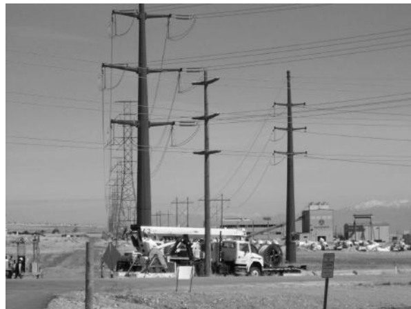
FIGURE 2.21 A 115 kV transmission line and a 345 kV transmission line with corner towers. (Courtesy of West Power Inc.)
