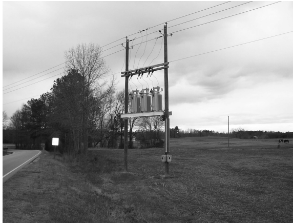
FIGURE 3.103 Photograph of three single-phase voltage regulators down-line on a distribution feeder.
