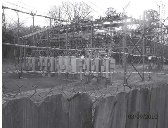
FIGURE 3.100 Photograph of single-phase voltage regulators on distribution feeders in the substation.
