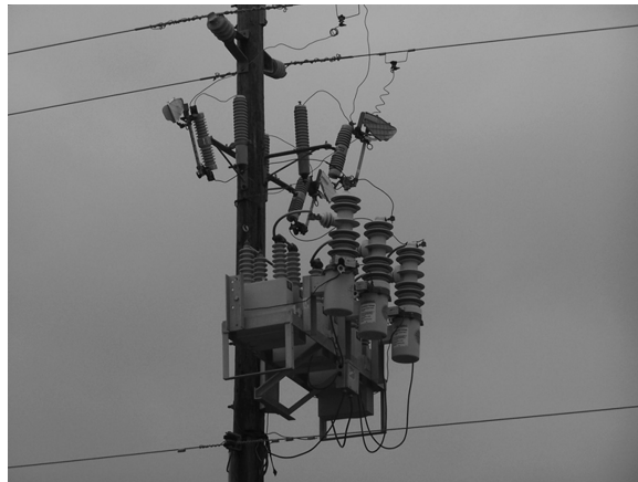
FIGURE 3.105 Photograph of a pole-top switched capacitor bank.
