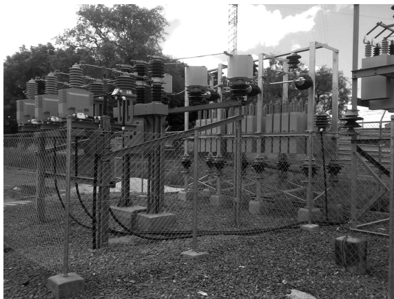
FIGURE 3.102 Photograph of a substation capacitor bank. (© Copyright 2012 Siemens. All rights reserved.)
