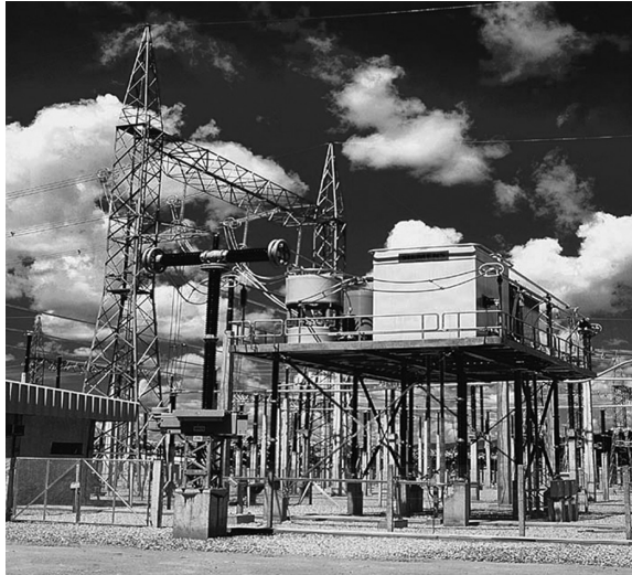
FIGURE 3.55 Photograph of a series compensation installation. (© Copyright 2012 Siemens. All rights reserved.)
