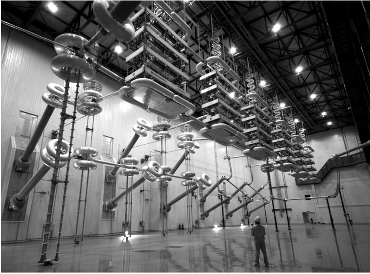
FIGURE 3.70 Conventional HVDC thyristor valve hall. (© Copyright 2012 Siemens. All rights reserved.)
