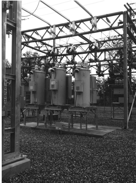
FIGURE 3.98 Photograph of three, single-phase bus voltage regulators.
