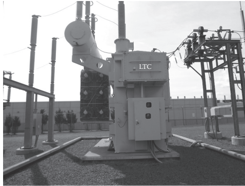
FIGURE 3.96 Photograph of a distribution substation power transformer with an LTC.
