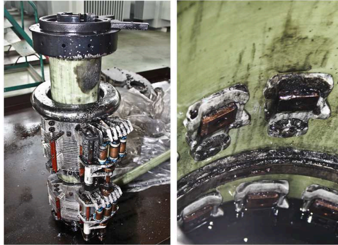
Fig. 2 The contactor in the On-load voltage regulating switch barrel and the switch
