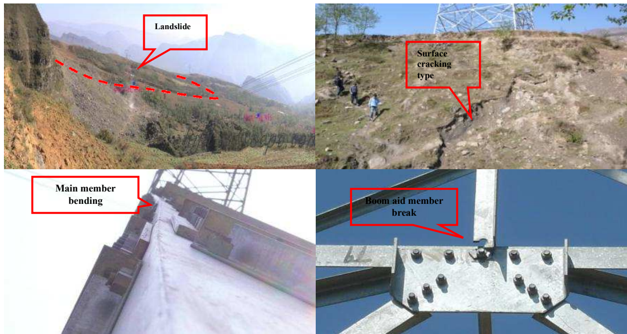
Figure 1 Impact on transmission lines by the resurrection of ancient landslides
