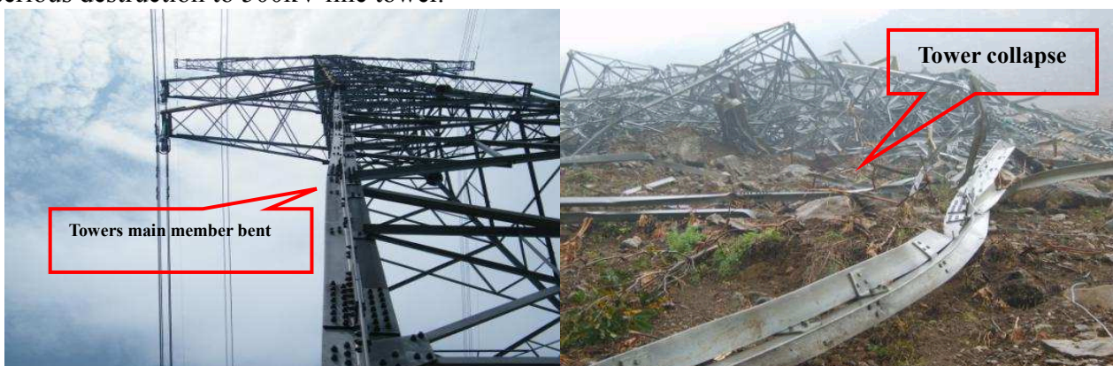
Figure 2 Impact of landslide for 500kV transmission line
