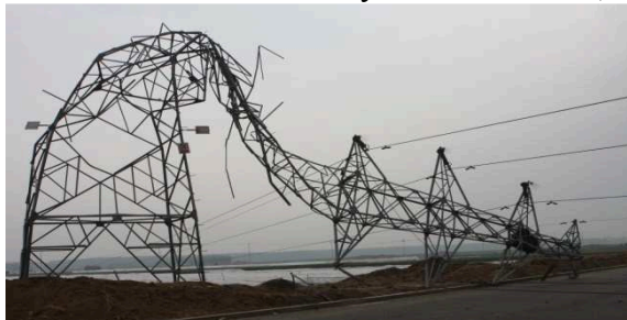
Fig.1 A case of #12 tower failure for 110 kV transmission line
