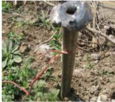
Figure 3 The connection of original grounding with lead wire
