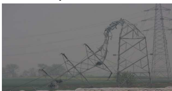
Fig.2 A case of No.13 tower failure for 110 kV transmission line
