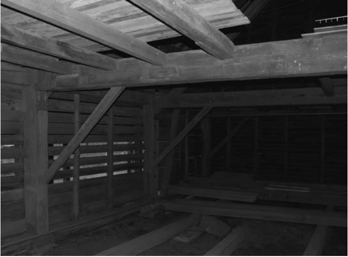
Figure 4.2 Timber beam in historic barn, Cane River Creole National Historical Park, Natchitoches, Louisiana
