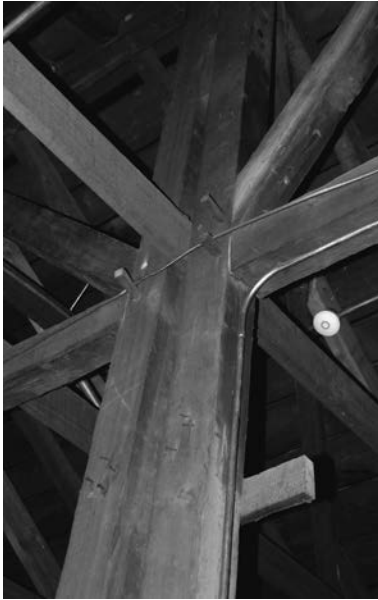
Figure 6.1 Timber column in historic barn, Cane River Creole National Historical Park, Natchitoches, Louisiana
