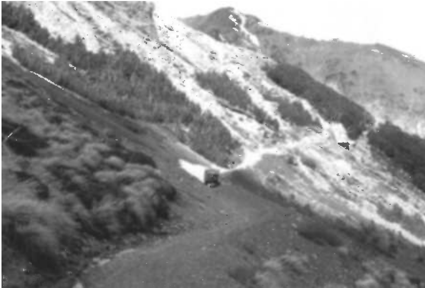
Fig. 8.7. Mass erosion associated with a backcountry road into a nordic ski area. South Island, New Zealand.
