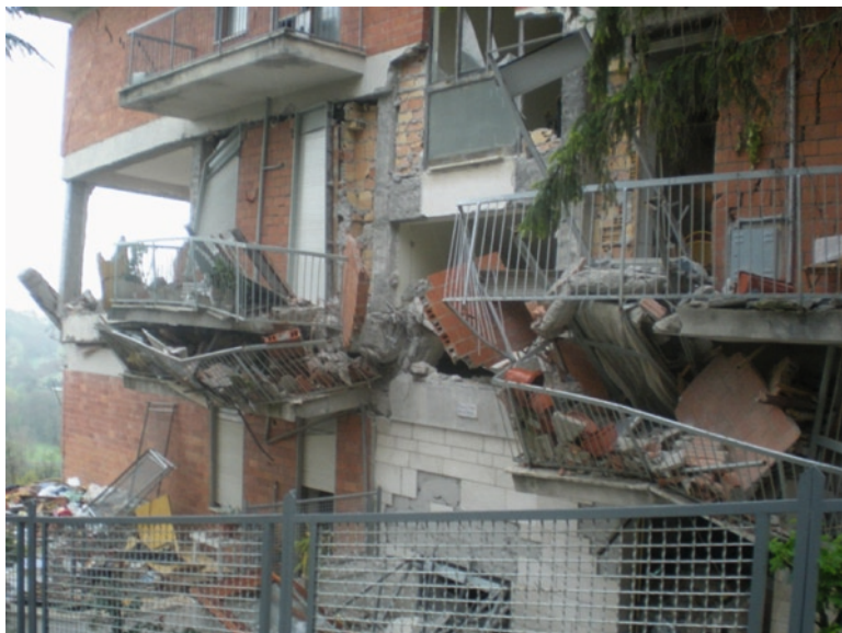
Fig. 13.7 L'Aquila city: reinforced concrete (RC) frame building that has suffered mid-floor compression
