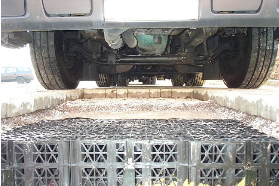
Figure 10.2 A contaminated field car park showing oil staining on permeable blocks and on the gravel bedding layer (reproduced by permission of Tim Puehmeier).
