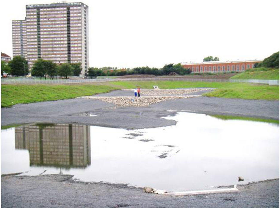
Figure 27.2 A new SuDS pond under construction on the south side of Glasgow (courtesy A. Duffy).
