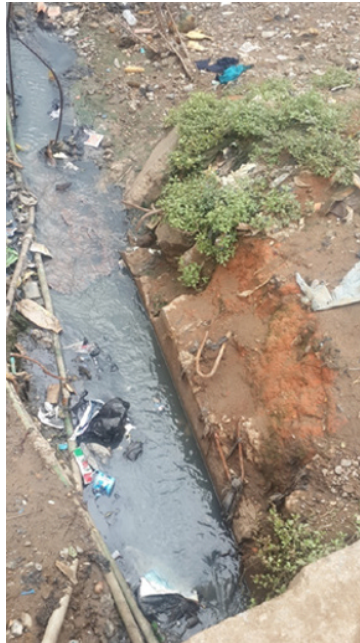
Figure 22.1 Blocked drainage system in Ijora, Lagos State, Nigeria.
