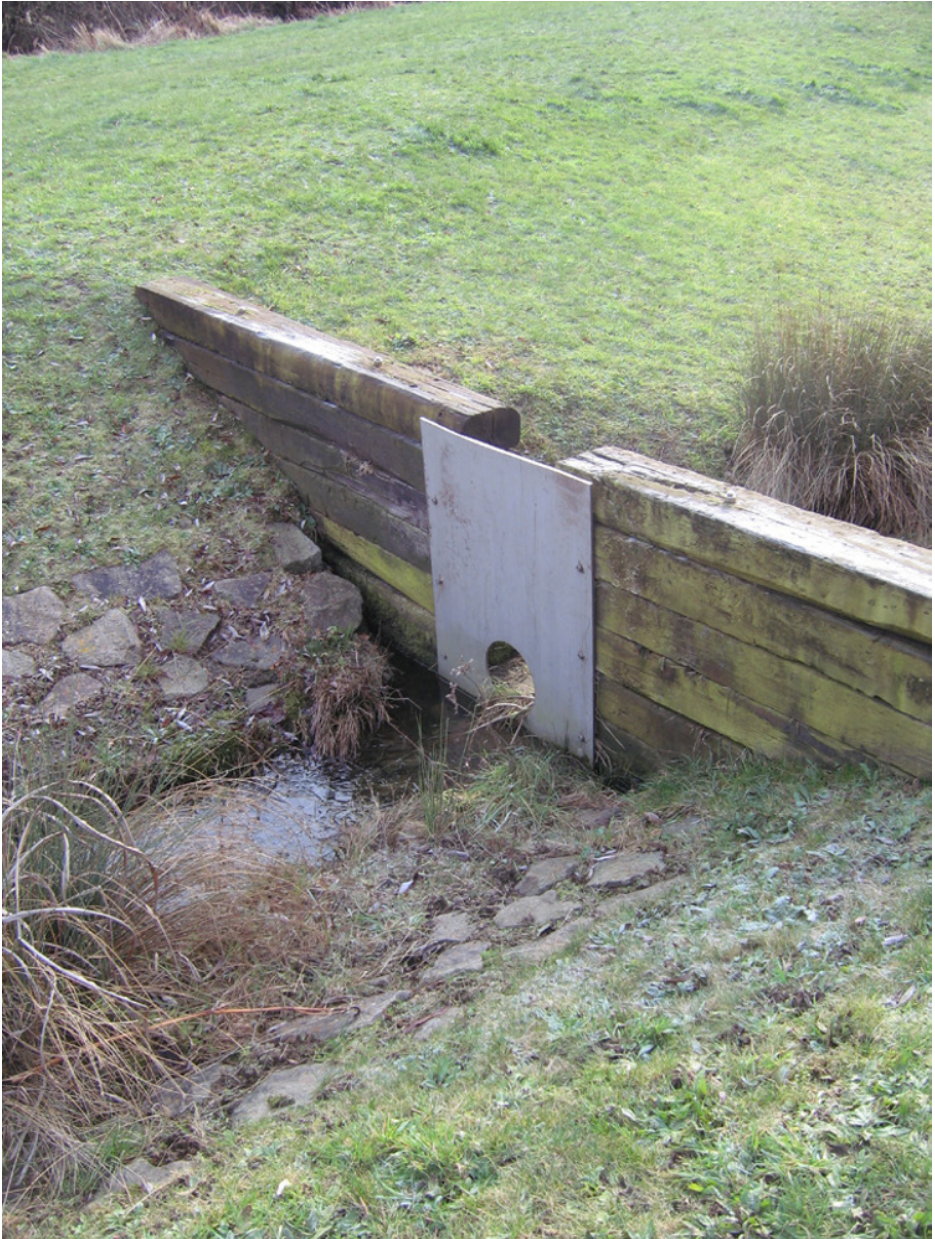
Figure 5.9 Weir at the SuDS management train in Hamilton, Leicester, UK.
