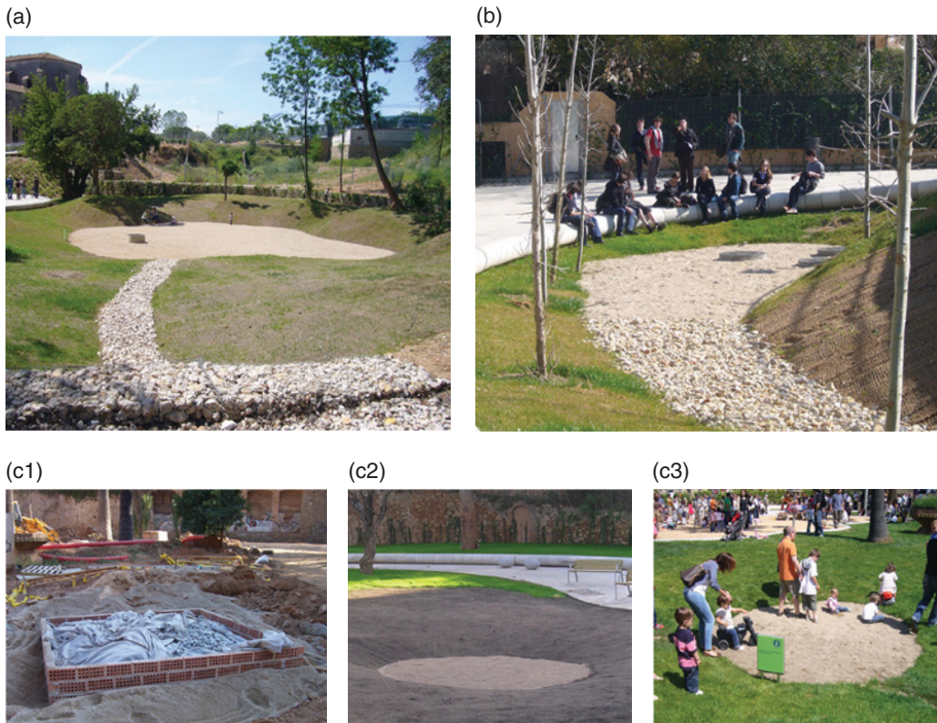
Figure 26.5 (a) Filter drains and infiltration pond (b) Retention pond at the end of filter drains (c1) Starting of construction of infiltration well (c2) Finishing of infiltration well (c3) Infiltration well integrated in the park. (Photos courtesy of Roberto Soto of BAGUR SA).
