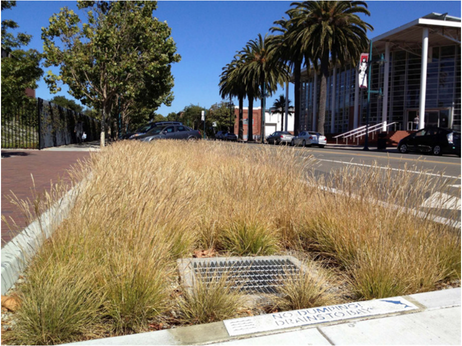
Figure 5.6 Bioretention system, installed in a central reservation, Emeryville, California, USA (freely available).
