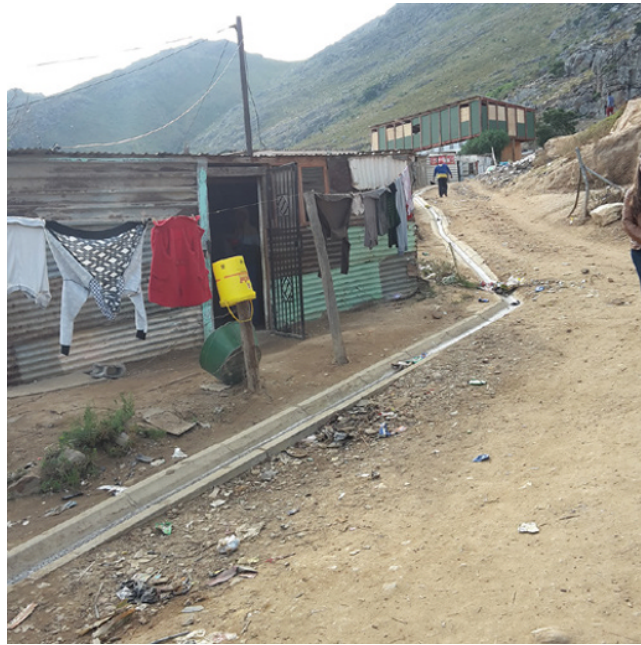
Figure 24.3 A drainage culvert alongside the road leading to the top of the settlement.
