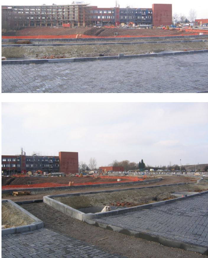
Figure 13.5 Three-storey office block at Stewartby, Bedfordshire, UK, showing the construction of the combined PPS/GSHP system.
