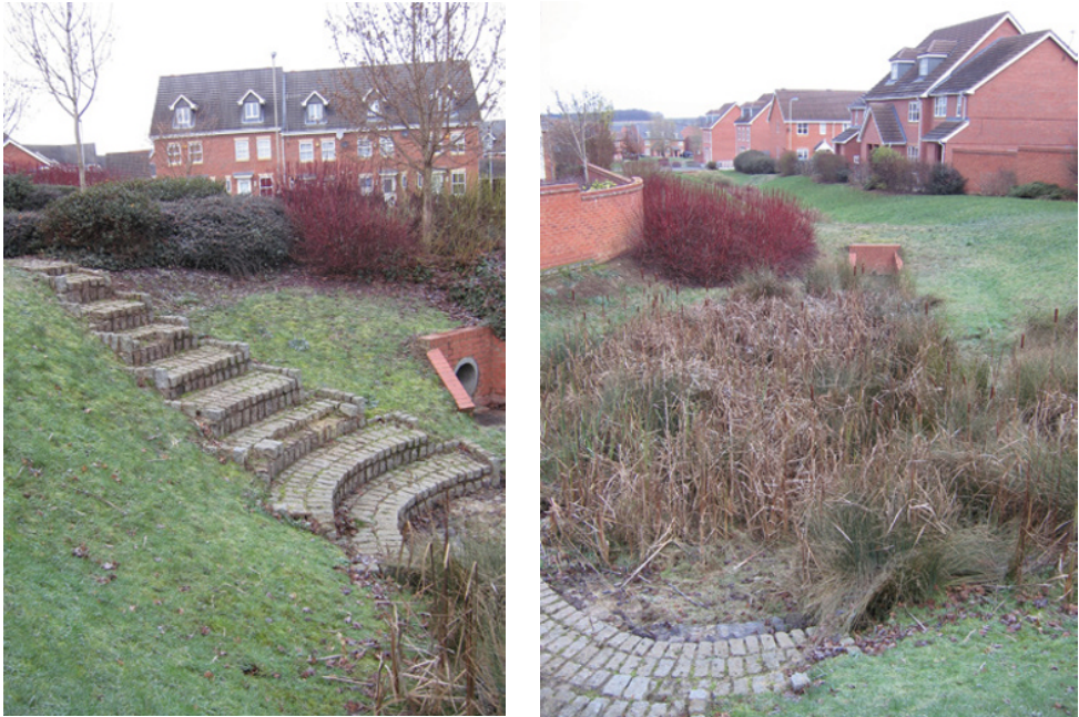
Figure 7.6 (left) Engineered feature leading down to (right) small wetland area, swale and filter strips, N. Hamilton, Leicestershire, UK.
