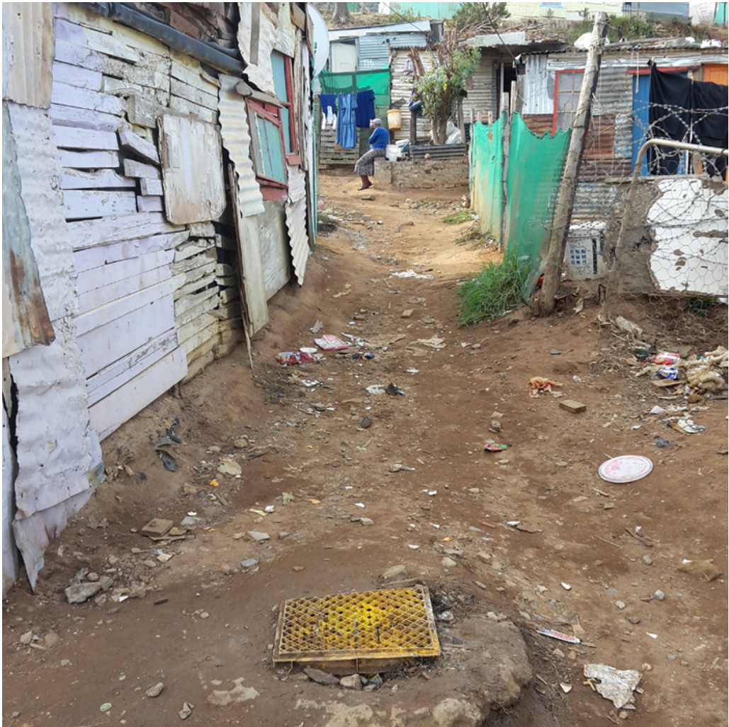
Figure 24.6 A community-led initiative to create a greywater discharge catchpit linked to a shallow pipeline.
