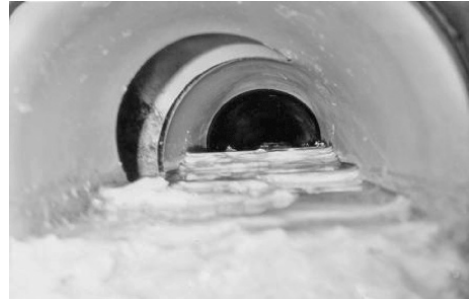
Figure 5-32 Sintering of a pipe invert.
