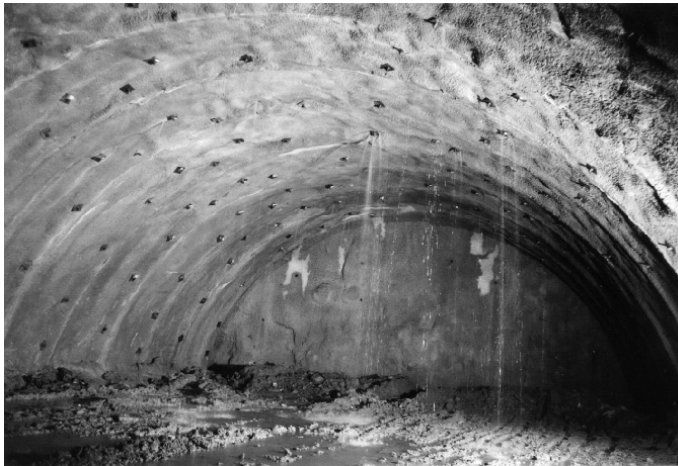
Figure 5-2 Water inflow at the face of the Schönrain Tunnel near Gemünden.
