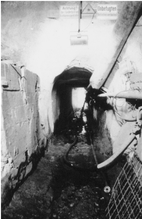
Figure 2-23 Abutment for bracing in a fault zone for the Mini-Fullfacer, Westtangente Bochum.
