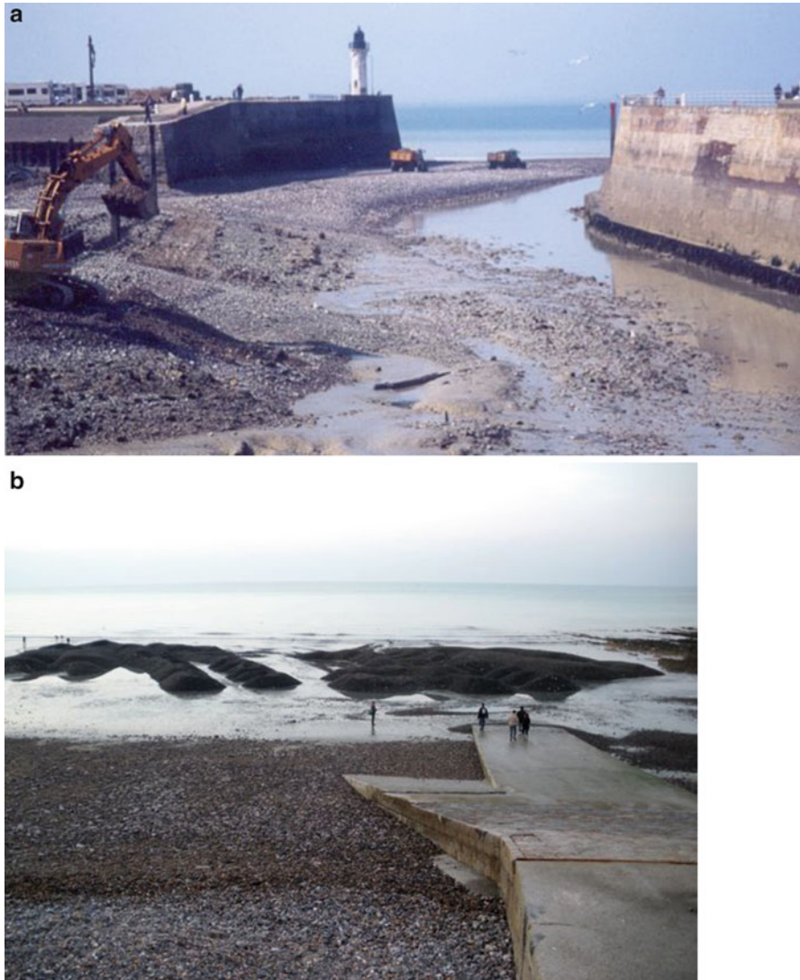
Fig. 6.14 Bypass system use along the Upper-Normandy coast. Dredging of the port of Saint Valéry-en-Caux (a) (Photo, Costa 1990). After dredging pebbles in the port fairways of Dieppe (cf. Fig. 6.13), deposition on the beach of Puy (Downstream of Dieppe Harbor) (b) (Photo, Authorities of Dieppe Harbor 2011)
