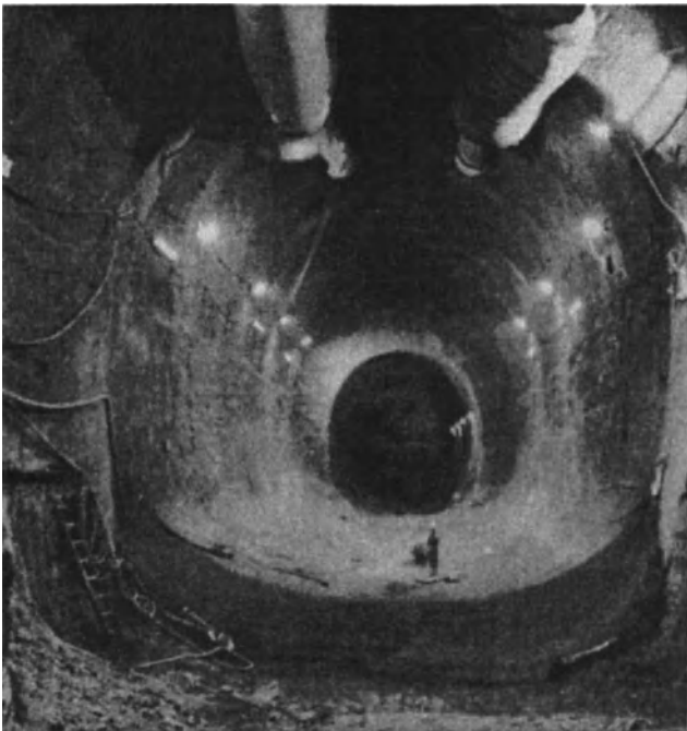
Fig. 11-6. Channel Tunnel. TBM Erection Chamber on UK shore. Excavated by Voest-Alpine AMT70 Roadheader in chalk.
