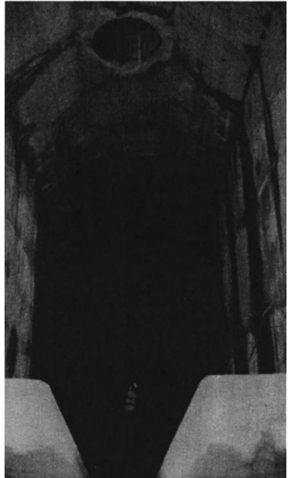
Fig. 15-4. D-4 drop shaft air-separation chamber, looking toward down-comer (note separate air vent in foreground).
