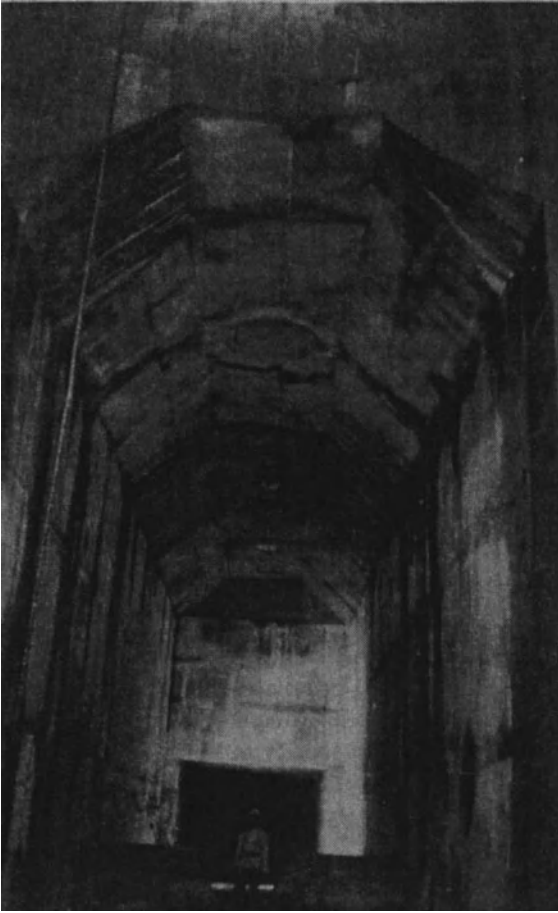
Fig. 15-5. D-4 drop shaft air-separation chamber, looking downstream toward exit conduit (note separate air vent).
