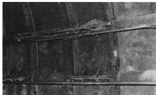
Fig. 3-36. Horizontal electrolevel beams (EI Beam Sensors) installed in BART subway tunnel to monitor vertical movement during tunneling operations for San Francisco Muni Metro Turnback Project.
