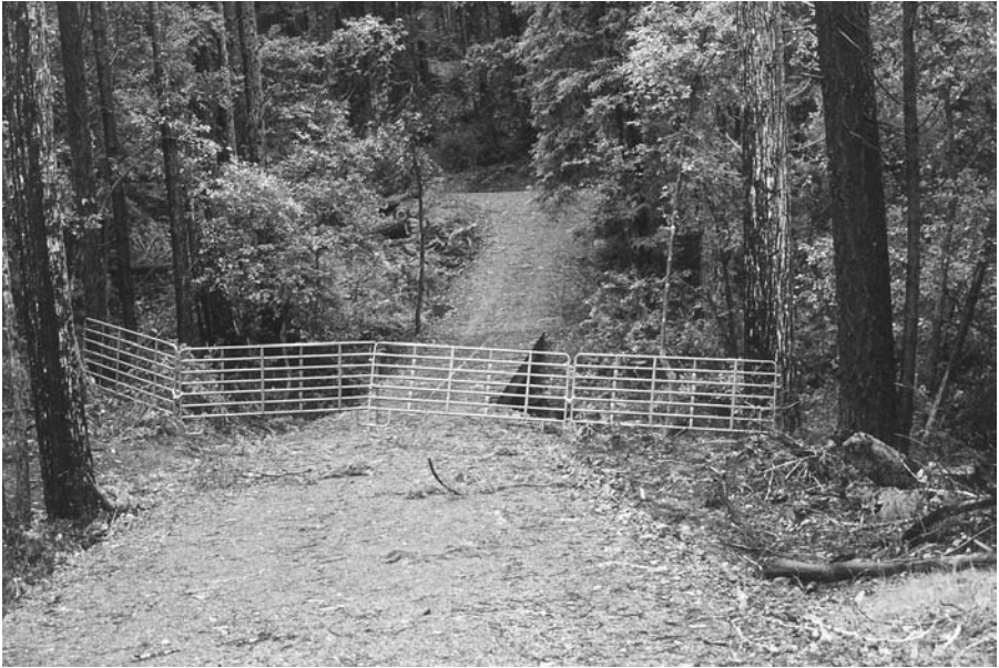
Photo 13 A controlled access road; note the well rocked road and bridge crossing, the latter taking the place of a culvert — Mendocino County, California. (Photograph by Walter Smith.)
