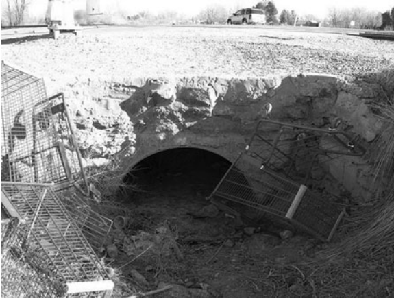
Figure 3-1. Example of Obstruction in a Culvert.
