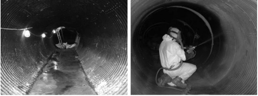
Figure 5-26. Left, Culvert Before Rehabilitation. Right, Spray-Applying of Polyurethane. Courtesy of Sprayroq, Inc.
