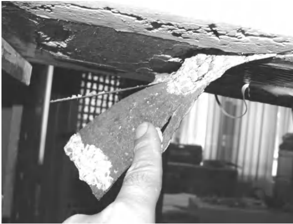
Figure 5 Plat end debonding in specimen C3I521
