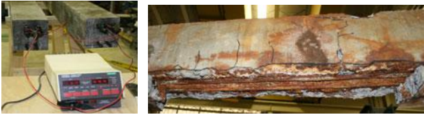
Figure 12 Test setup Figure 13 Typical deterioration
