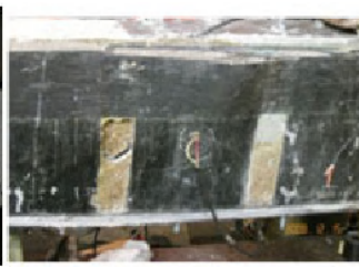
Figure 13 Shear failure of FRP-RC
