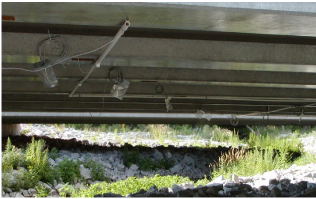
Figure 1 Mini-DIN plugs and PVC wire runs used in the field instrumentation
