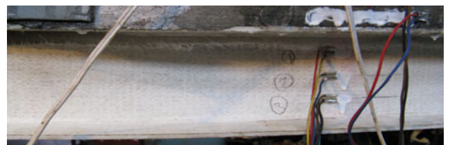
Figure 9 Failure pattern of FRP-concrete composite deck
