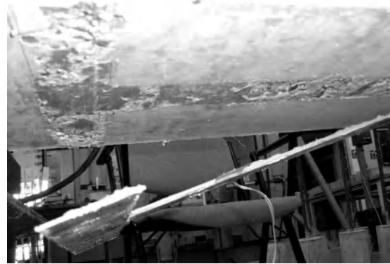
Figure 3 Delamination of the additional anchorage for B4
