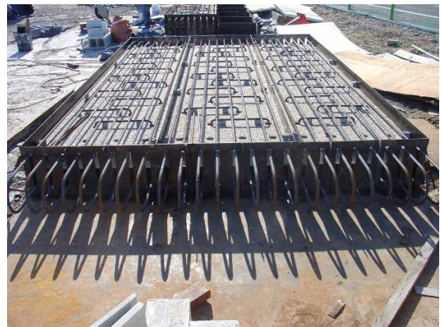
Figure 4 Fabrication of the precast FRP-concrete composite deck specimens (after assembling of rebars)
