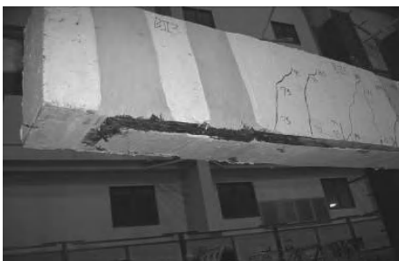
Figure 2 The end debonding failure picture
