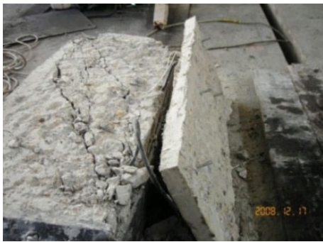
Figure 20 Failure of interfaces in L4
