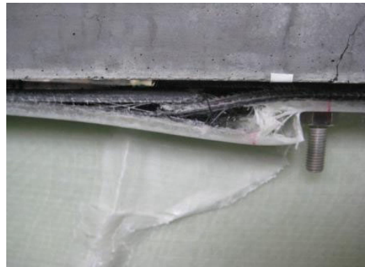
(b) HFRP flange delamination failure
