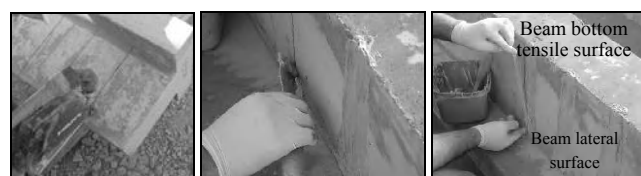
Figure 1 NSM technique with CFRP laminates for the shear strengthening of RC beams
