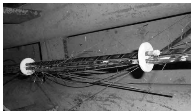
(b) Pull-off damage
