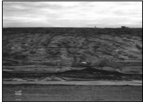
Fig. 17 Massive Soils Loss on Slopes
