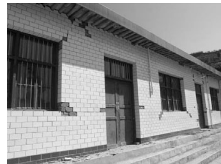
Fig. 5 Damages to brick-wood building in Haoping Village of Wudu District, Gansu Province(VIII degree)
