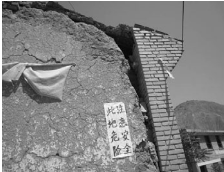
Fig. 7 Lengthways fracture on joint of the wall and brick column of Leiba Village hospital of Lixian County, Gansu Province.(VII degree area)
