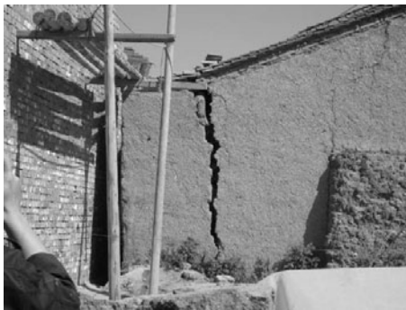
Fig. 8 Damage to the adobe-wood house at the Wudang Village of Zhangxian County, Gansu Province. (VI degree)
