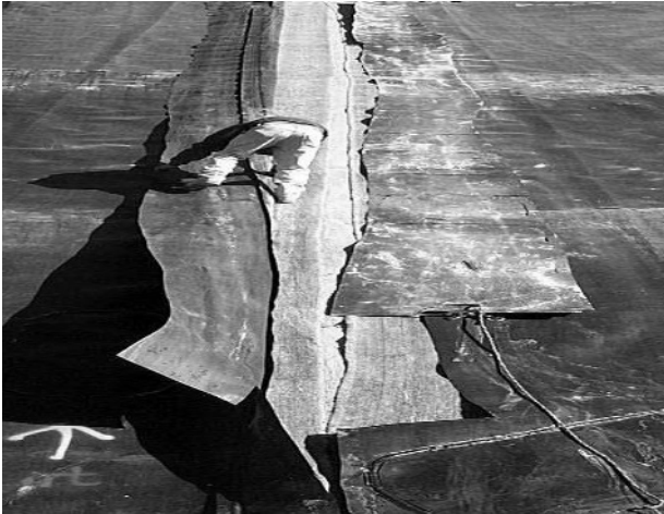
Fig. 7 Panel separation of a GCL in a composite liner in California (after Thiel and Richardson, 2005)
