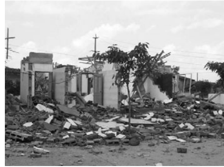
Fig. 2 A brick-wood house collapsed, Jiulongzhen Town, Mianzhu City, Sichuan Province. (IX degree)
