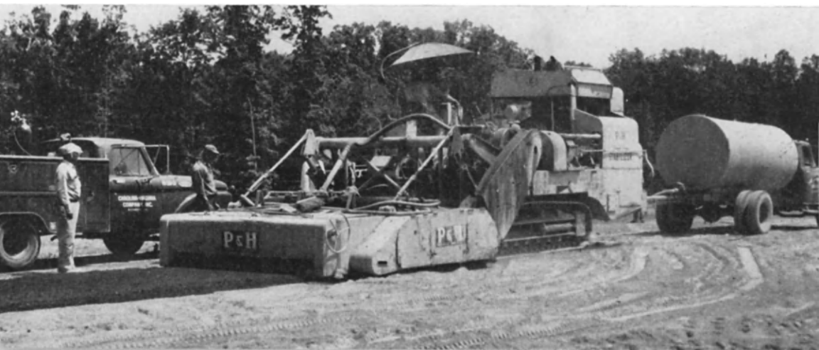
FIG. 49. A large output single-pass stabilising machine constructing a sub-base for a concrete road. Cement is spread on the formation in advance of the machine and water is supplied by a linked bowser.
