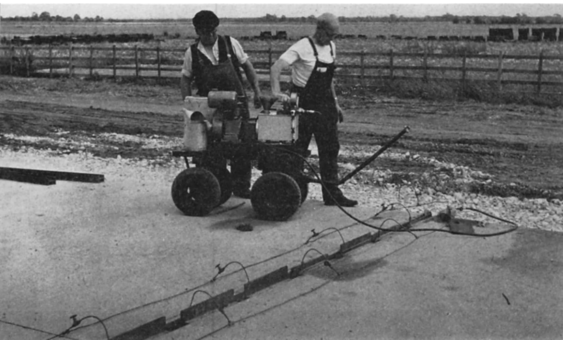
FIG. 62. Jacks being inflated to prestress concrete road slabs at Winthorpe, Nottinghamshire. On completion of jacking, the joint is blocked and the jacks removed.
