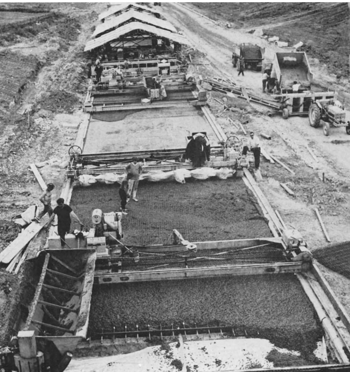
FIG. 32. A concrete train constructing reinforced concrete slabs, the concrete being side fed from the adjoining carriageway.
