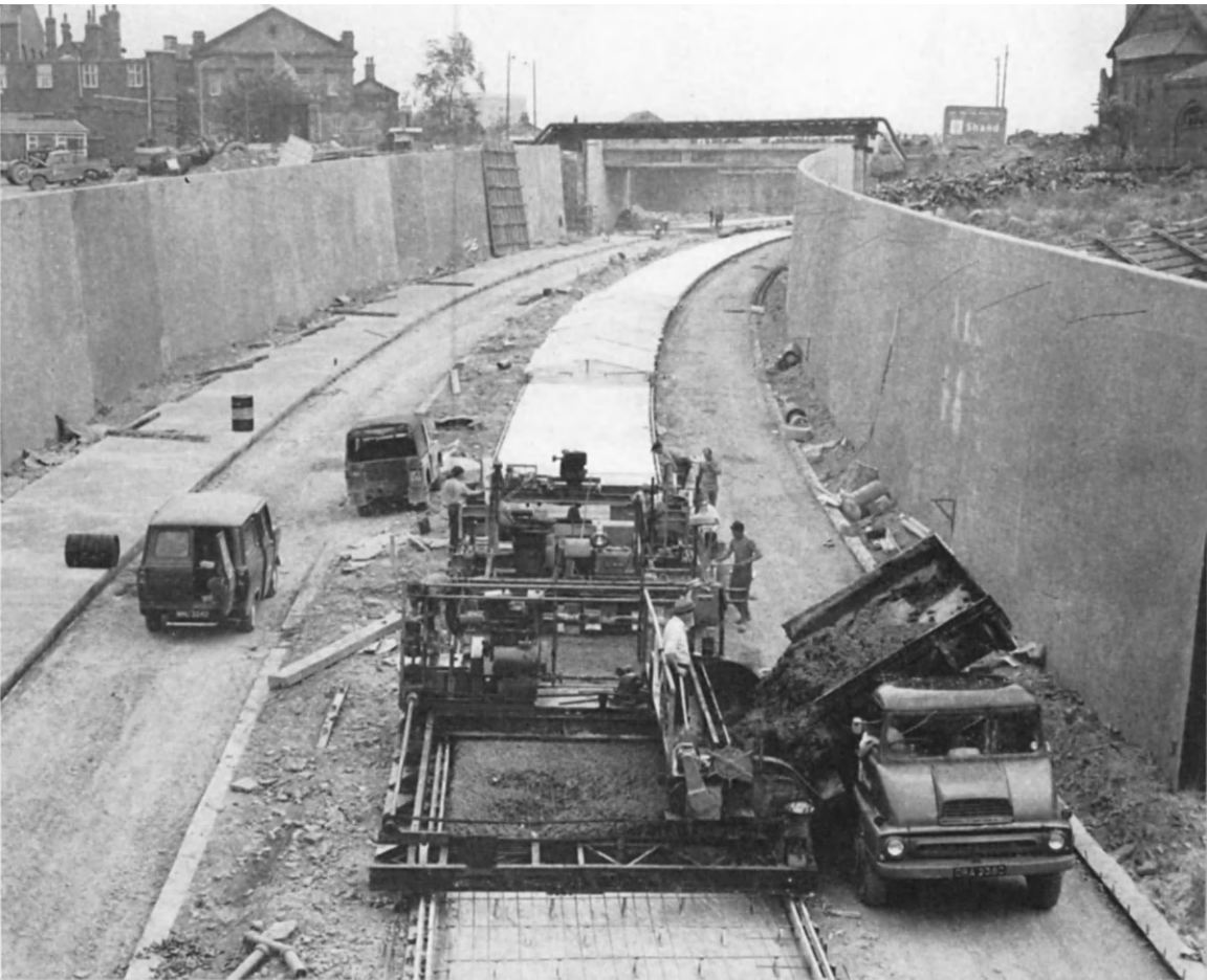
FIG. 33. A concrete urban motorway under construction by fully mechanised methods. Bar reinforcement supported on stools is being used.
