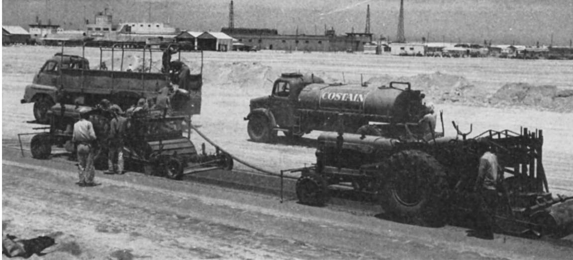
FIG. 48. Single-pass soil-cement equipment on airfield construction. Note the bagged cement supply to the cement spreader incorporated in the front machine with the water spray system fed from the bowser. The rear machine is a dropping weight compactor.
