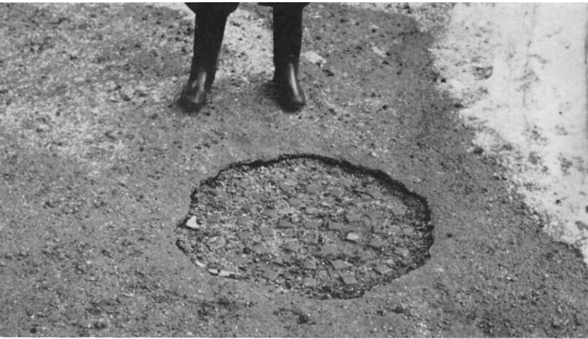
FIG. 12. Frost heave in a flexible pavement constructed on a chalk subgrade. The manhole cover has remained at the original level.
