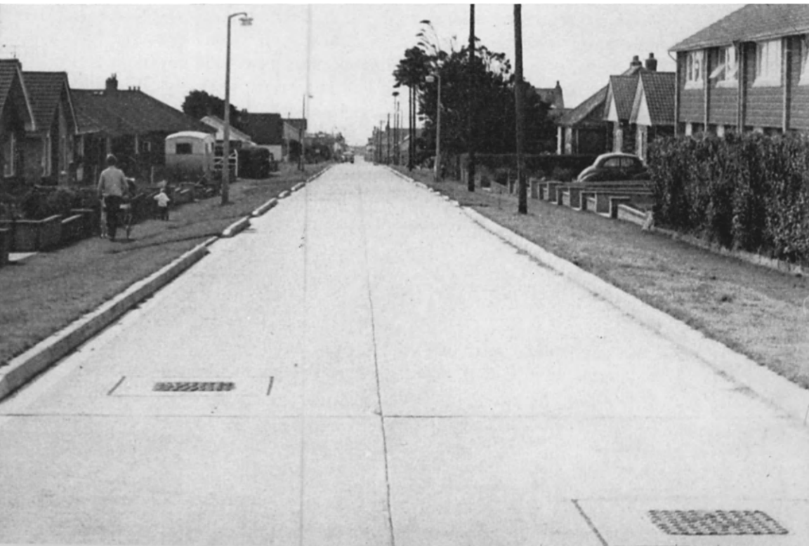
FIG. 22. Boxing out of gullies and manhole covers in separate slabs. Note the well sealed joints.
