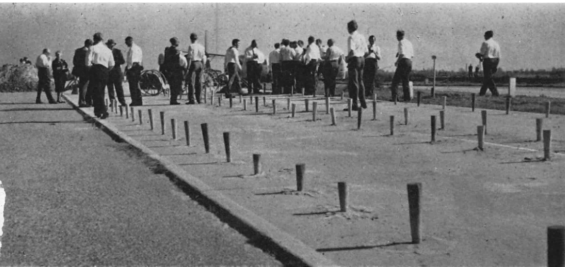
FIG. 68. Lifting of concrete slabs on a motorway. Cement grout is injected into holes drilled through the slab, the process being done in stages.
