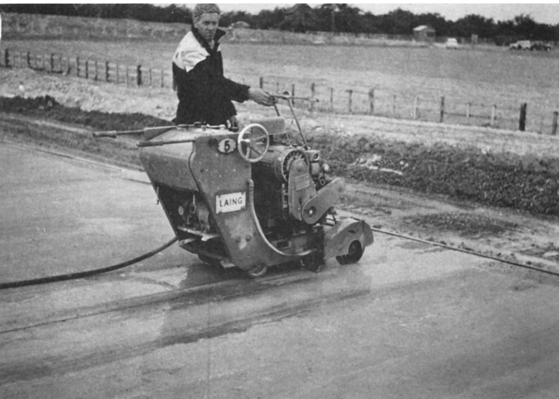
FIG. 21. A semi-automatic concrete saw cutting a contraction joint groove in hard concrete.
