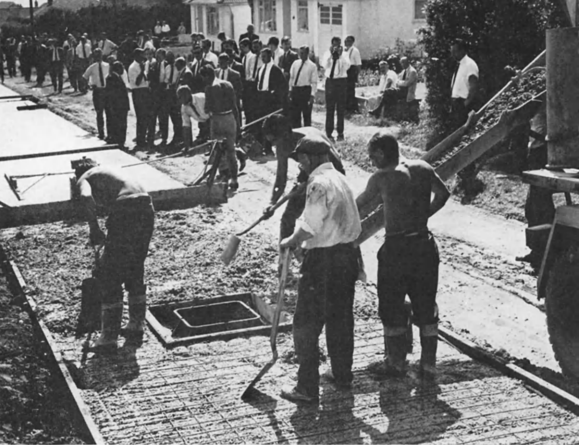
FIG. 17: A small concrete job in progress using ready mixed concrete. The base course concrete and reinforcement have been placed in the foreground and the top course is now being spread and compacted. Note the boxing out around the manhole cover.
