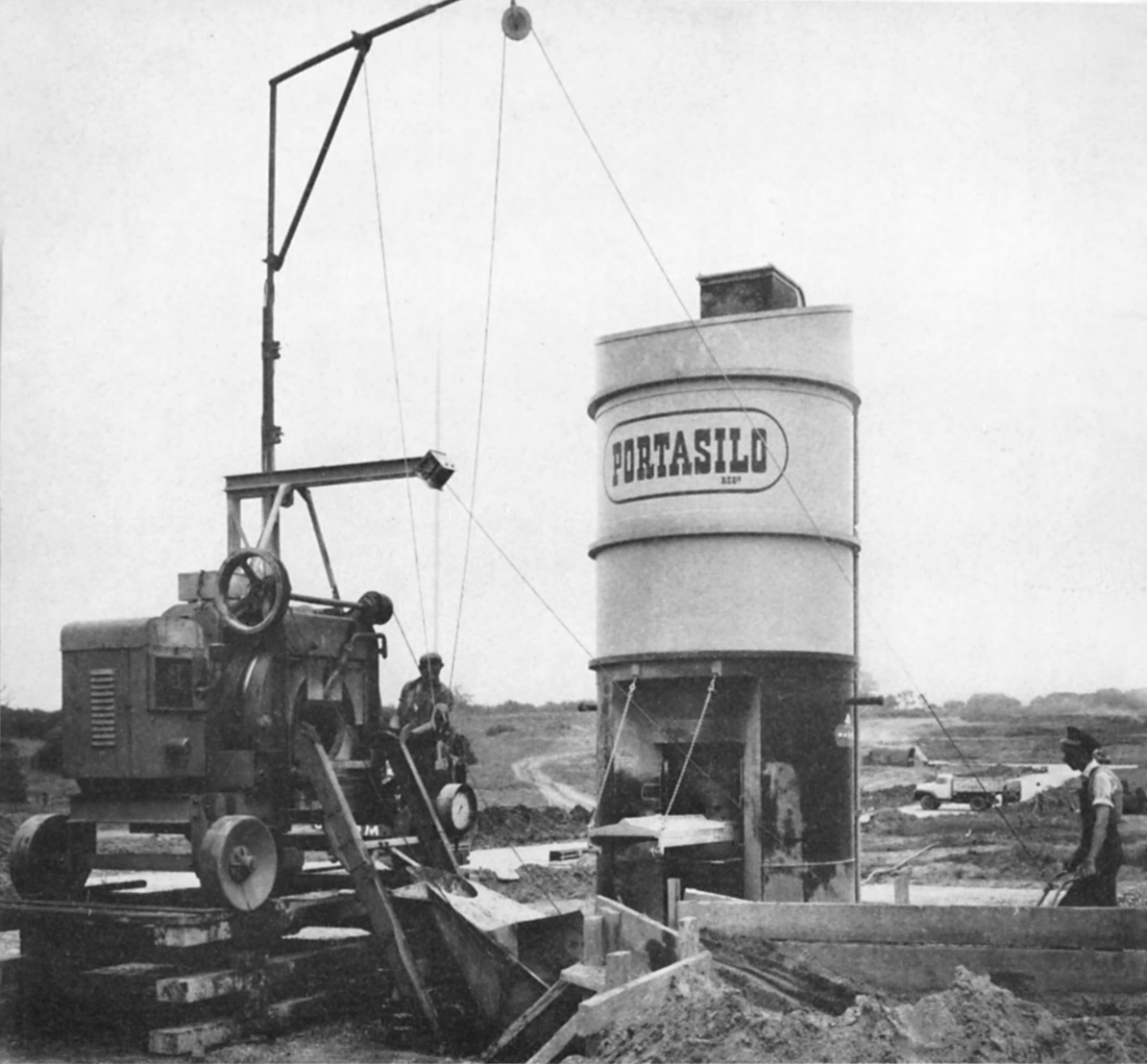
FIG. 16. Concrete batching and mixing plant showing cement silo, weighbatching equipment and timber separating walls between different aggregate sizes.
