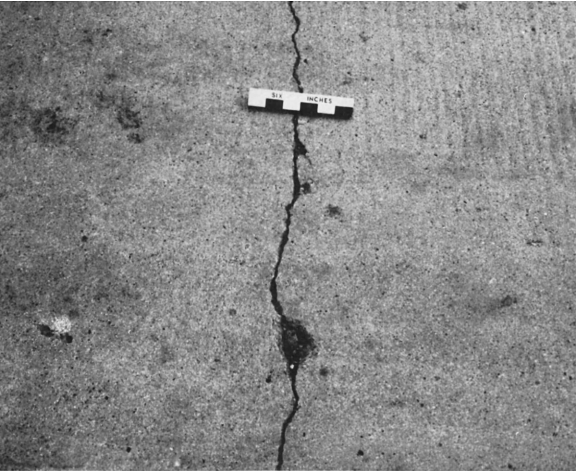
FIG. 5. A crack in an unreinforced concrete slab showing excessive width and incipient deterioration due to edge spalling.
