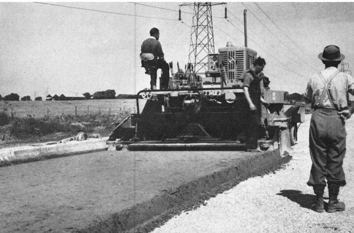
FIG. 53. Laying lean concrete using a bituminous paver to form the base for a motorway.
