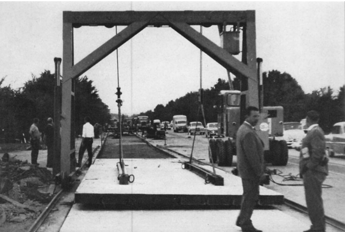
FIG. 69. A precast prestressed concrete slab about 40 ft \times 11 ft being lifted into position on a German motorway to replace a 25-year-old defective section.
