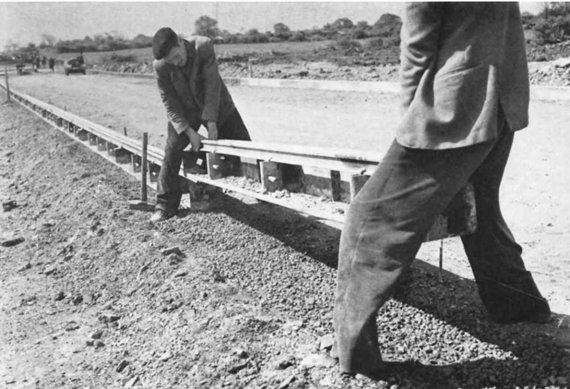
FIG. 28. Laying a heavy duty form used for fully mechanised construction on a bed of plastic fine concrete.
