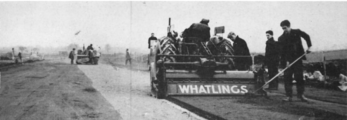
FIG. 47. A cement spreader (background) and single-pass machine mixing cement into soil to produce a soil-cement sub-base for a motorway.
