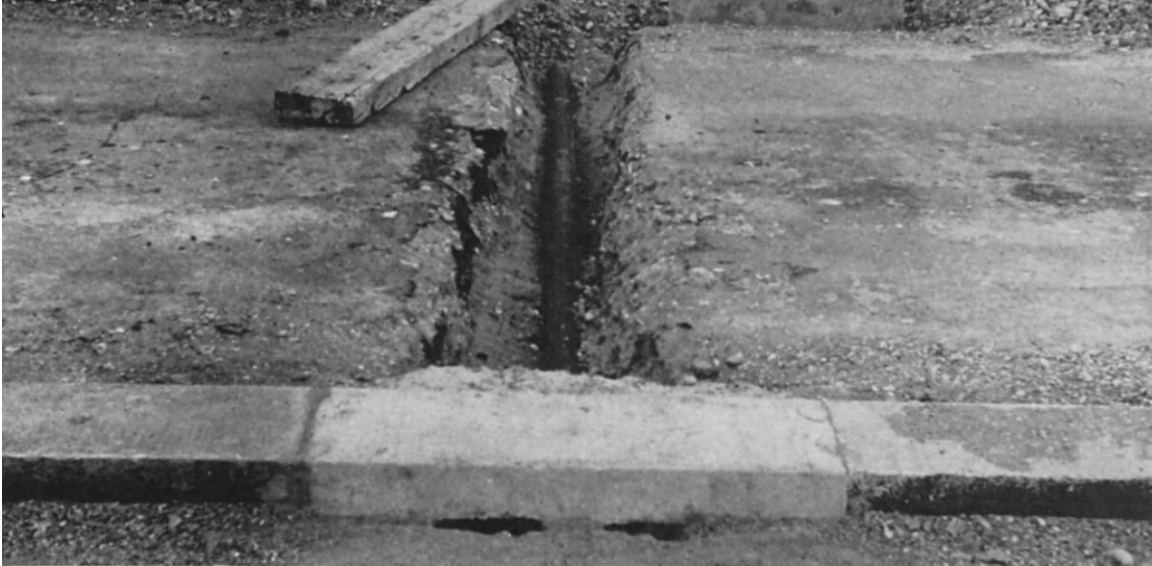
FIG. 11. Drainpipe laid in hard shoulder to dispose of surface water trapped on top of cement stabilised base prior to surfacing. Note entry holes for water in kerb.
