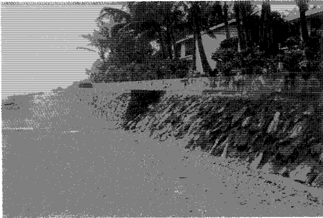
Plate 5. Seawall along the front of a south-coast tourist resort, Vitilevu Island, Fiji. Although effective in preventing shoreline erosion at this particular spot, the building of the seawall has caused a lot of scour of beach sand resulting in the exposure of beach rock at several points.
