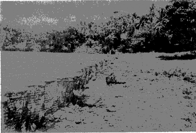
Plate 4. Coastal protection at Kumi Village, Vitilevu Island, Fiji consists of a line of oil drums filled with rocks and cemented together. The drums rust and fall apart after a while. The sea washes over the seawall and contributes to its undermining.
