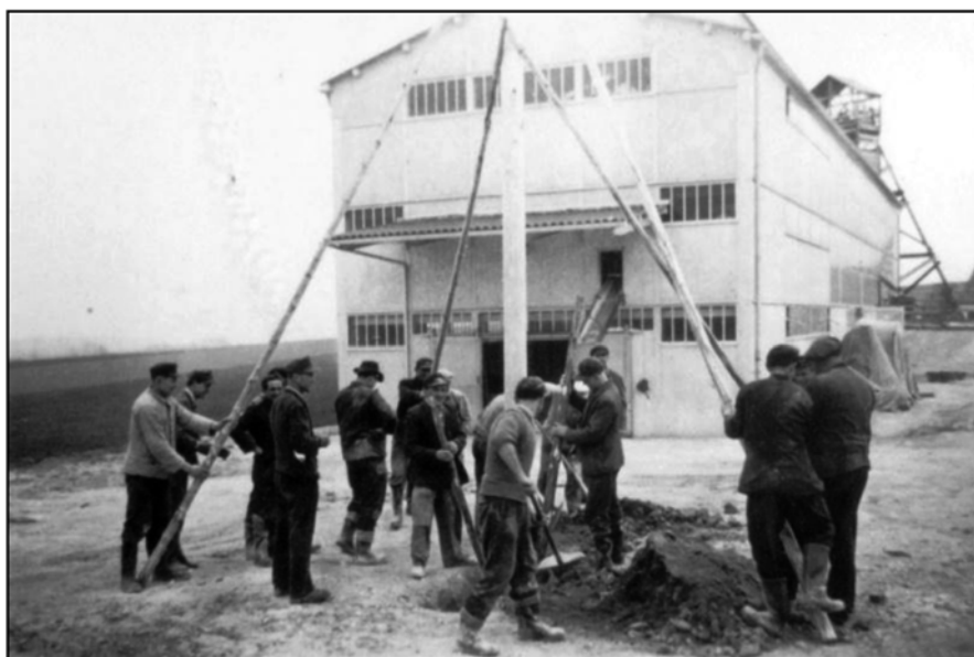
Fig. 1.4k Making the ball mill near the open pit operational. In the background the head frame of the old shaft is visible
