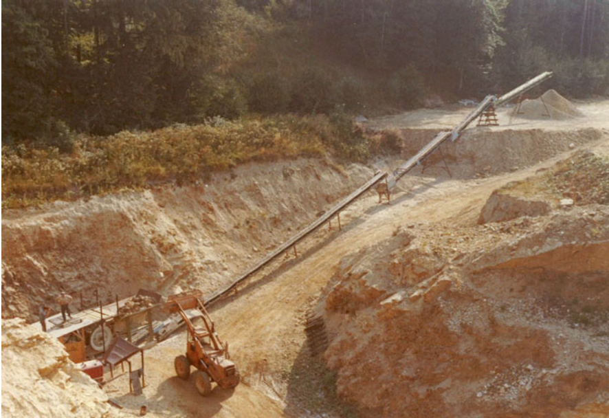
Fig. 1.6c At an advanced level the feldspar has been transported with a front-end loader from the working site in the open pit to the crusher. The pre-treated raw material is transported out of the mine by a staircase-like set of conveyor belts (Courtesy of Gottfried Feldspat GmbH)
