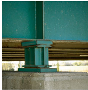
The rocker support for this bridge girder allows horizontal movement so the bridge is free to expand and contract due to a change in temperature. (5)
