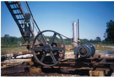
Flat or V-belts are often used to transmit the torque developed by a motor to a wheel attached to a pump, fan or blower.
