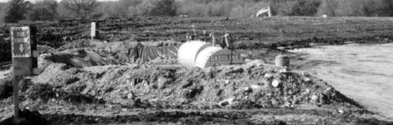
FIGURE 11.1 On-site fuel facility.
