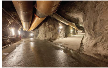
Figure 3. Access to excavation front with concreted sills (Source: Venda Nova III Constructor).
