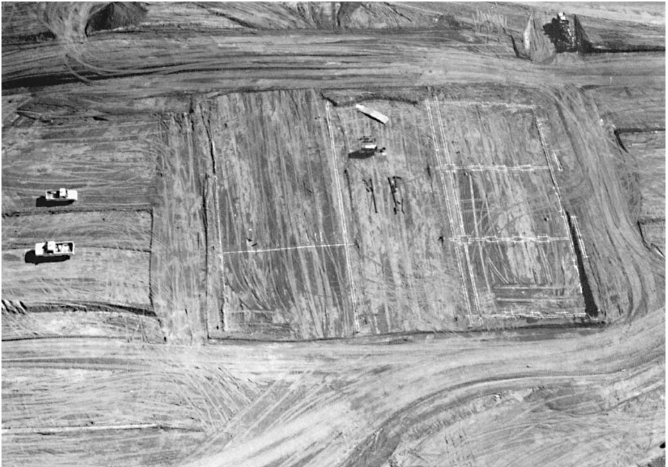
Figure 9.33 Chalking for foundation layout. (Courtesy of AVCO Community Developers, Inc., and Mann Theatres Corporation of CA.; William Boggs Aerial Photography. Reprinted with permission.)
