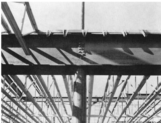
Figure 14.10 Main steel floor beam and column with joist hangers. (Courtesy of Westmount, Inc., Real Estate Development, Torrance, CA; William Boggs Aerial Photography. Reprinted with permission.)
