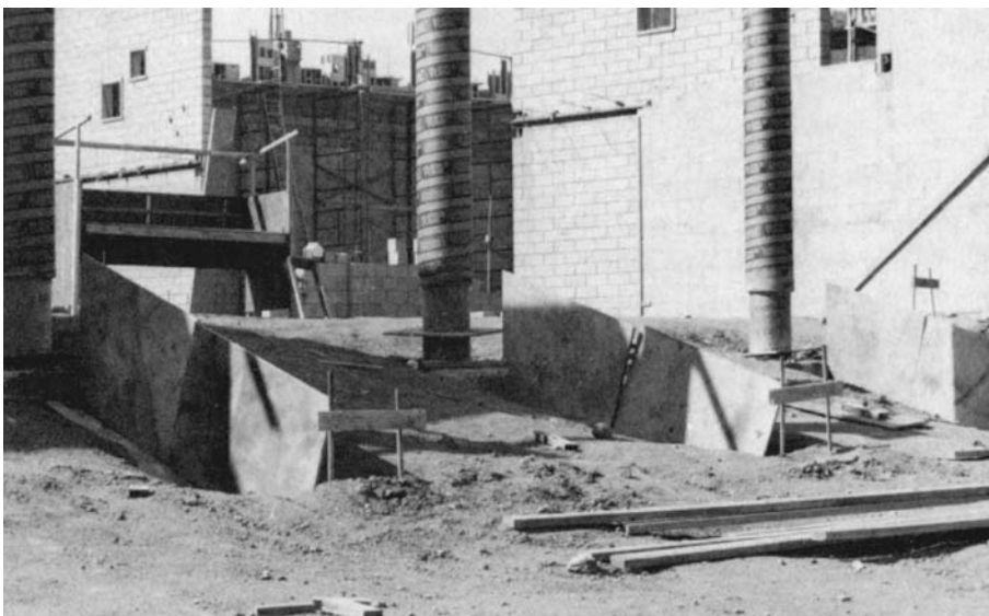
Figure 19.19 Columns to support upper floor and forms for the stairs adjacent to the handicap ramps.
