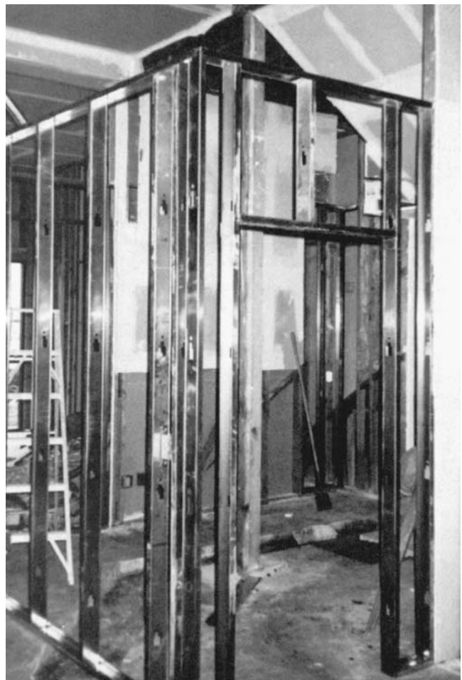
Figure 21.15 Wall framing—steel studs. (Reprinted by permission from The Professional Practice of Architectural Working Drawings , 2d Ed., © 1995 by John Wiley & Sons, Inc.)
