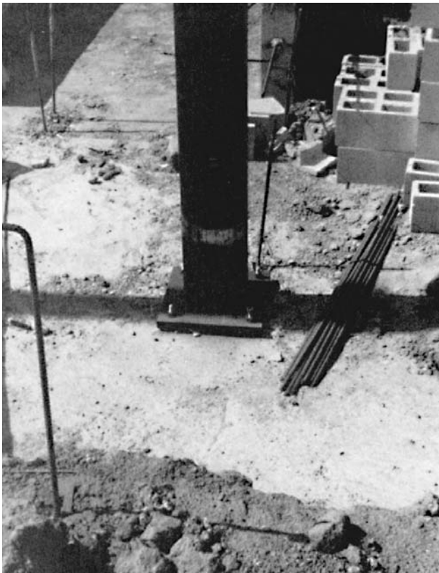
Figure 9.38 Steel column on concrete pad.
