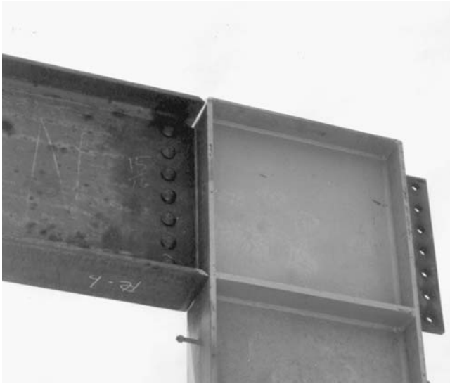
Figure 7.26 Photograph similar corner-column and beam connection. (Courtesy of Rich Development.)
