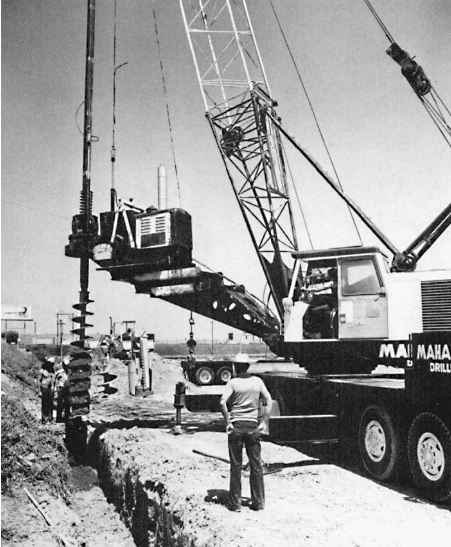
Figure 9.40 Drilling holes for concrete caissons. (William Boggs Aerial Photography. Reprinted with permission.)
