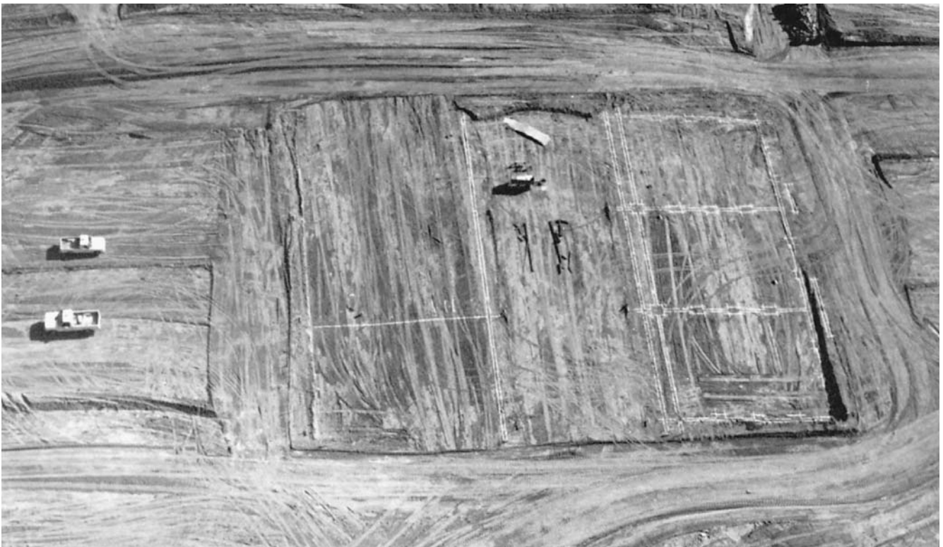
Figure 19.16 Chalked lines ready for trenching. (William Boggs Aerial Photography. Reprinted with permission.)
