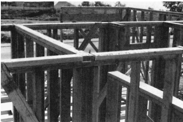
Figure 10.19 Intersection of interior walls at the top plates. (Courtesy of William F. Smith—Builder.)
