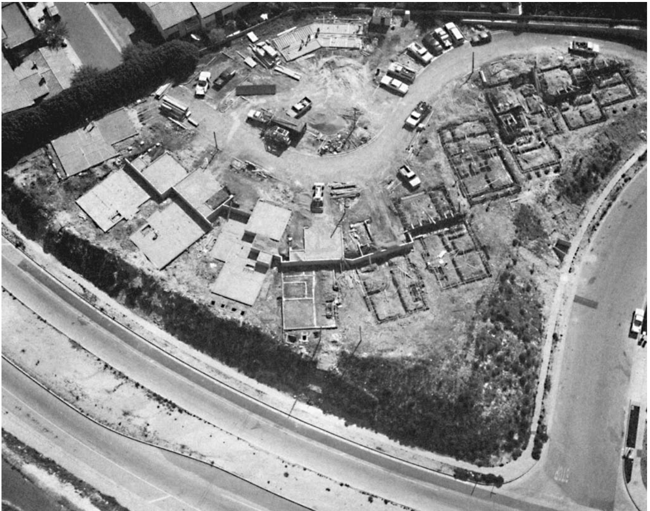
Figure 9.43 Foundation trenching—poured concrete floor and foundation. (Courtesy of William F. Smith—Builder; William Boggs Aerial Photography. Reprinted with permission.)
