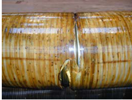
FIGURE 5.4 Internal Sheath Crack. Source: O'Brien [7]. (For color version of this figure, the reader is referred to the online version of this book.)
