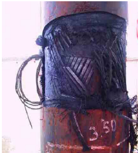
FIGURE 5.8 Corrosion of Armor Wire. Source: Boschee [11]. (For color version of this figure, the reader is referred to the online version of this book.)
