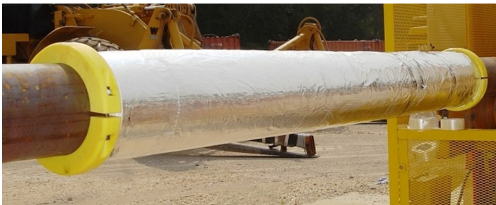
Figure 17.6 Centralizer and insulation material flowline.
