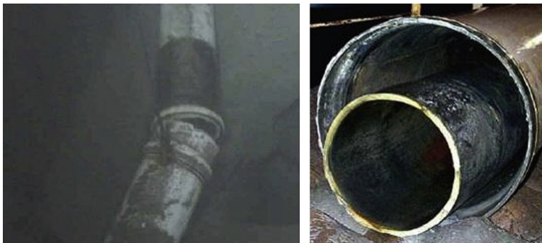
Figure 10.1 Pipelines that failed due to fatigue damage.
