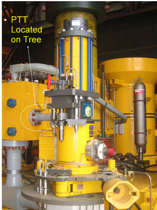
Figure 22-38 PTT Located on a Subsea Xmas Tree
