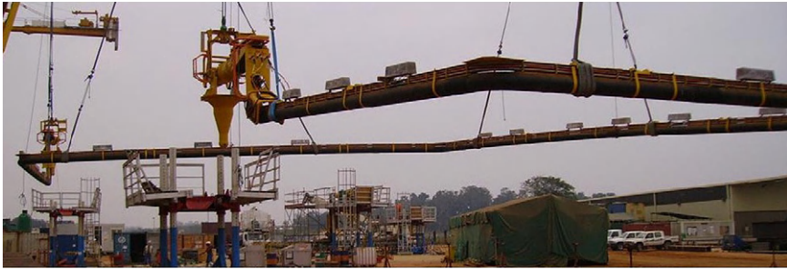
Figure 21-4 Well Pu-PG to Manifold Jumper [2]
