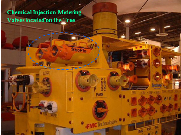
Figure 22-40 Chemical Injection Point at Tree (Courtesy FMC Technologies)
