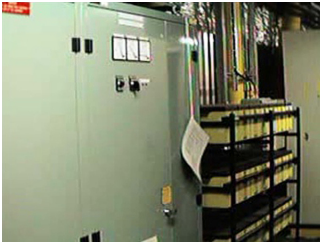
Figure 8-5 UPS and Battery Rack
