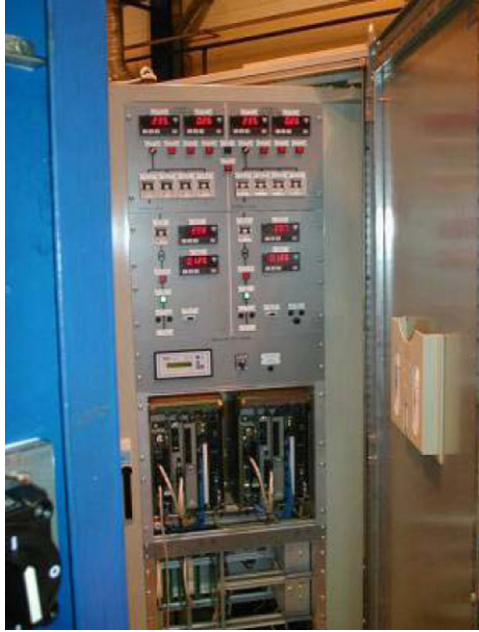
Figure 7-10 Electrical Power Unit (EPU)
