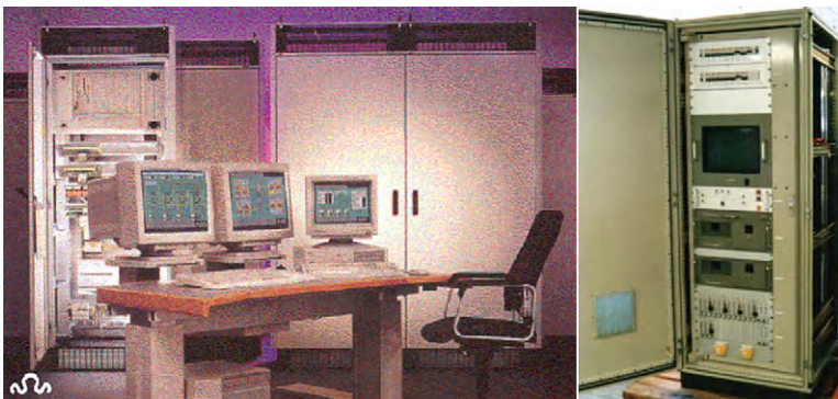
Figure 7-8 Mater Control Station (MCS)
