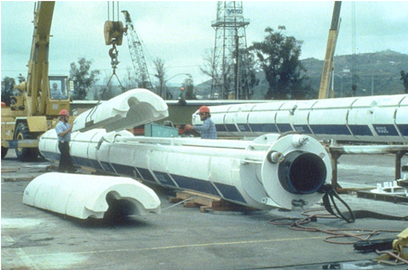
Figure 26-17 Typical Buoyancy Modules
