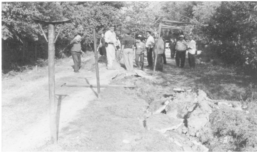
Figure 3: Surface break in Gölcük displacing posts by 4 m during the 17 August earthquake.
