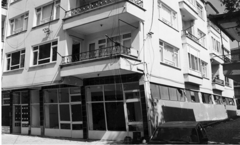
Figure 7: Reinforced concrete frame structure in Yalova which displayed first story column-hinge deformation, but did not collapse after the 17 November earthquake (grade of damage 5 – class of vulnerability D).
