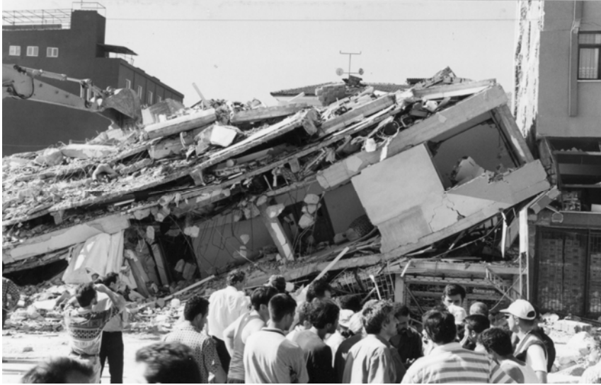
Figure 5: Reinforced concrete frame structure that collapsed in Gölcük after the 17 August earthquake (grade of damage 5 – class of vulnerability D).
