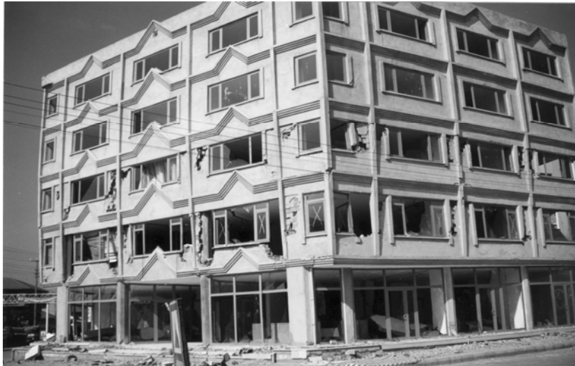
Figure 8: Reinforced concrete frame structure at Gölcük which displayed light structural damage but heavy damage to the infill brick walls after the 12 November earthquake (grade of damage 5 – class of vulnerability D).
