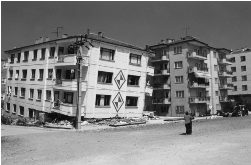
Figure 6: Reinforced concrete frame structure that sustained collapse of ground floor in the area Gölcük – Degirmendere after the 17 August earthquake (grade of damage 5 – class of vulnerability E).
