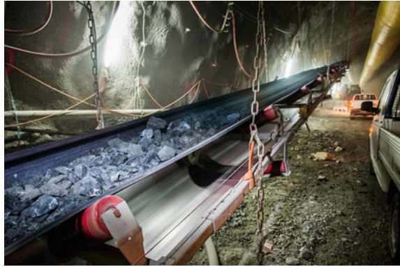
Fig. 19.10 Conveyor belt was used in Norway 14.3-km-long Solbakk tunnel (Reproduced from Ref. [5] by permission of TunnelTalk)
