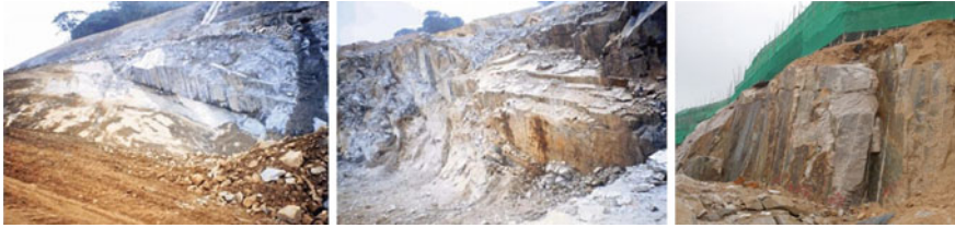
Fig. 1.41 Slope failure by discontinuities
