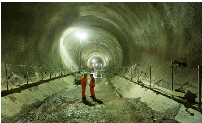
Fig. 21.41 A second mass-pass-transit cross-rail line in London lined with shotcrete Source www.theguardian.com/uk/crossrail
