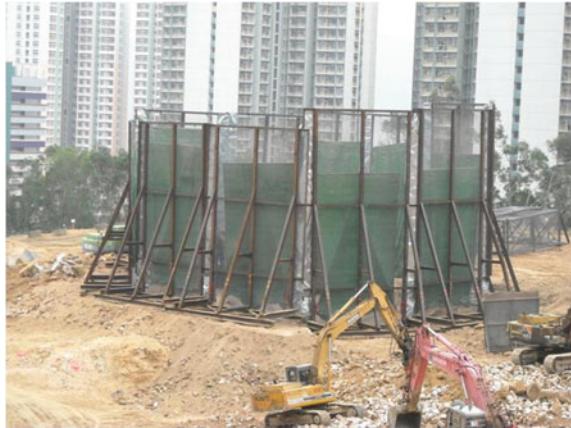
Fig. 11.34 Vertical screens covered with canvas as sound barriers are surround the blasting area
