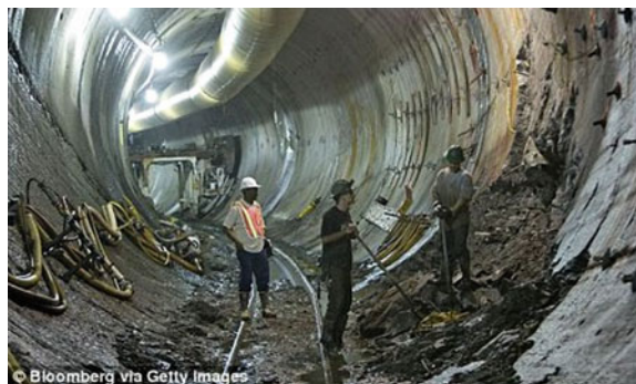
Fig. 1.43 Rock sliding failure from sidewall. 2001, East Side Access project in New York ( www.dailymail.co.uk/news/ )
