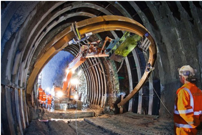
Fig. 21.43 The old steel arches of Holme Tunnel were replace with new arches Source www.railmagazine.com
