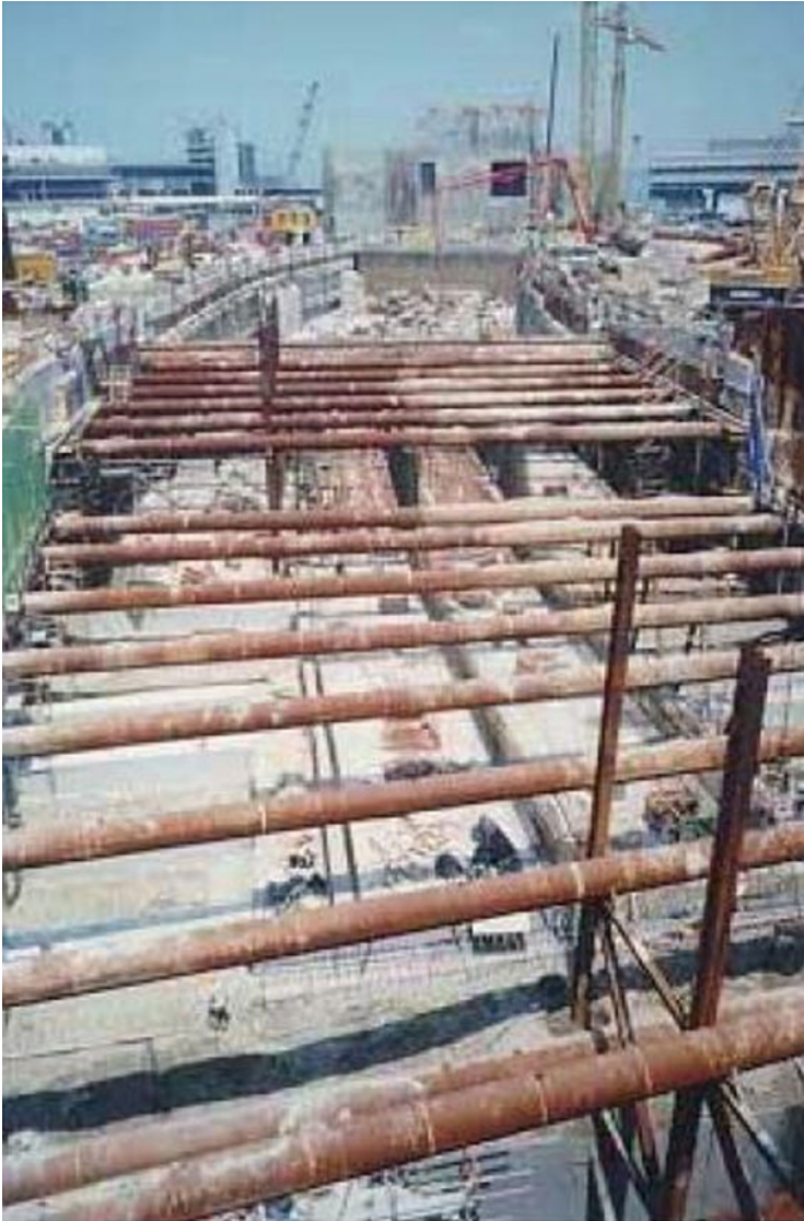
Cut and Cover Tunnel for the Airport Railway at the Central Reclamation in Hong Kong in Late 1996. Section of the tunnel pit formed by diaphragm wall and strutted by the use of steel tubes. The construction of the tunnel sections using in-situ method can be seen inside the pit.
