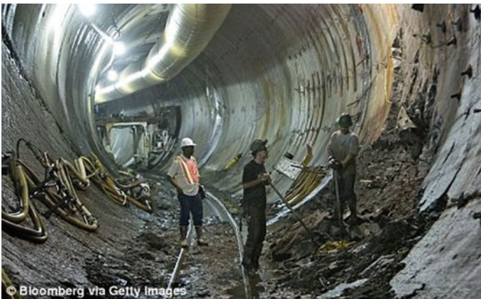
Fig. 23.3 Michael O'Brien (not in picture) died after a rock hit his head while he was working on the East Side Access Project in New York, 2011 (Source www.dailymail.co.uk/news/ )
