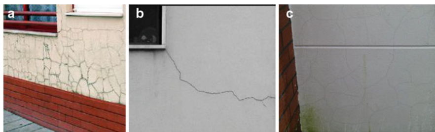
Fig. 2.30 (a) Mapped cracking/fissures; (b) oriented cracking in traditional render [71]; (c) cracking in pre-dosed render [65]
