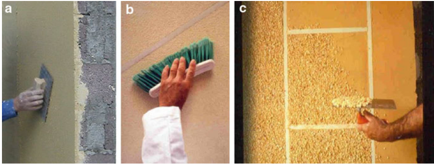
Fig. 2.27 (a) Execution of scraped finish: floating and (b) scrubbing; (c) application of finish in stone in pre-dosed renders [64]
