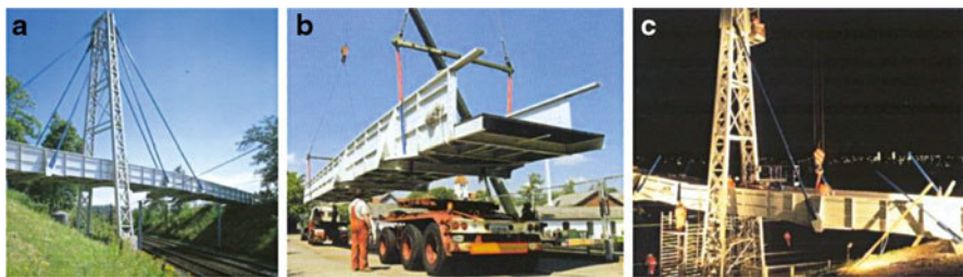
Fig. 11.25 The Kolding bridge: (a) general view, (b) transport of a 27 m long bridge segment and (c) bridge installation during the night [12]
