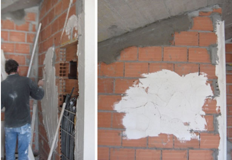
Fig. 3.19 Mechanical treatment of the substrate, eliminating warping and filling cavities with gypsum paste [25]
