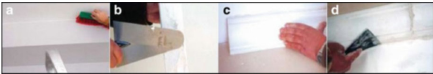
Fig. 3.51 Execution detail of a coving: (a) cleaning the substrate; (b) applying the gypsum, gluing over the decorative element with a trowel or a spoon; (c) manual pressing and slight movement of the piece in order to guarantee a good bond between the coving and the substrate; (d) elimination of the excess material and smoothing of the surface with a trowel [31]
