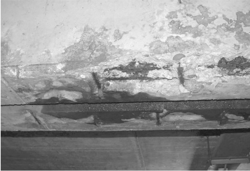
Fig. 4.14 Concrete degradation due to corrosion of reinforcements
