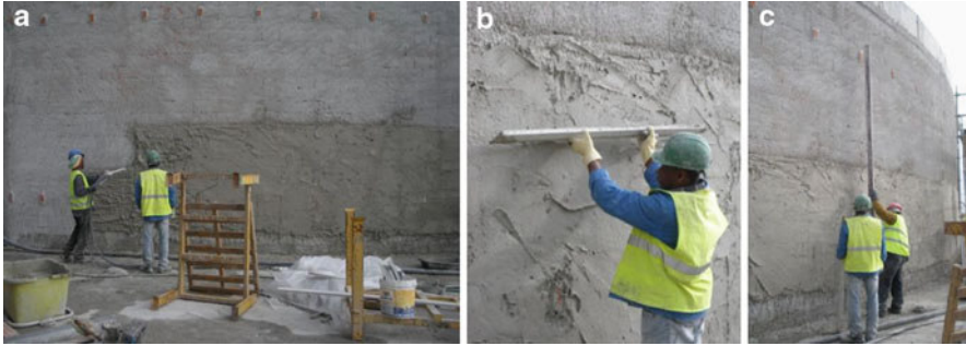
Fig. 2.25 (a) Application of the base coat with spraying device, reference points; (b) pressing and smoothing/levelling the mortar's coat; (c) checking the render's verticality with a reference support [67]
