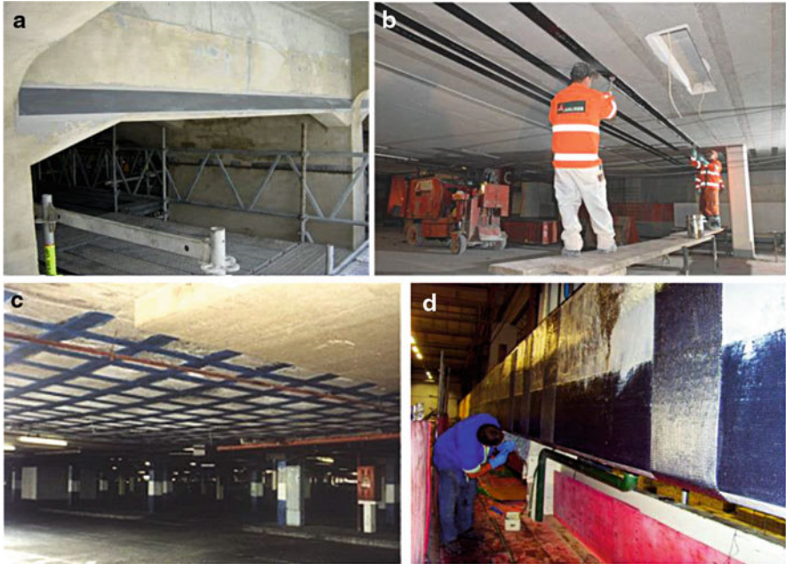
Fig. 11.37 Flexural strengthening of (a) beams, (b) slabs with strips, (c) slabs with sheets and (d) flexural and shear strengthening of a beam with sheets (adapted from [55, 10, 9, 58])
