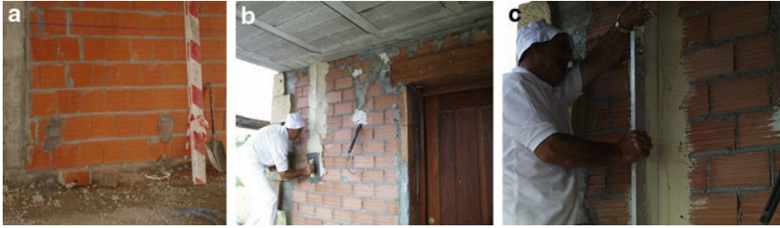
Fig. 2.24 (a) Points and lines technique for rendering mortars: masonry points in masonry before the application of interior plaster; (b) execution of a mortar line; and (c) checking its verticality with a bubble level [64]
