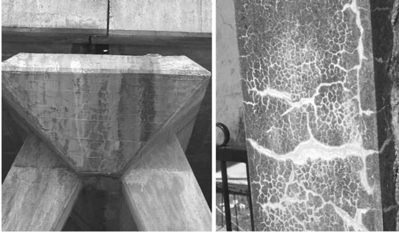
Fig. 4.15 Cracking caused by alkali-silica reactions
