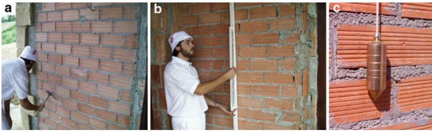
Fig. 2.21 (a) Removal of protrusions; (b) checking planeness with a ruler; and (c) verticality with a plumb line [64]
