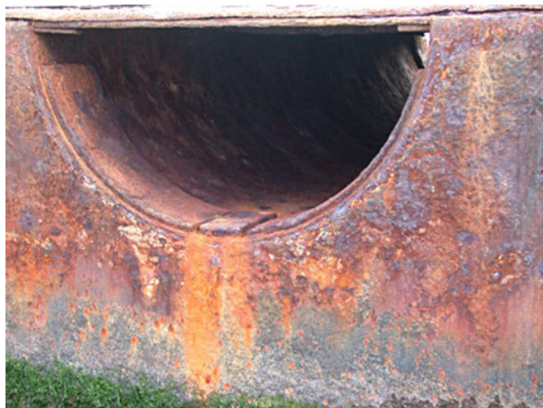
Fig. 15.5 Example of uniform corrosion (photograph by the author)
