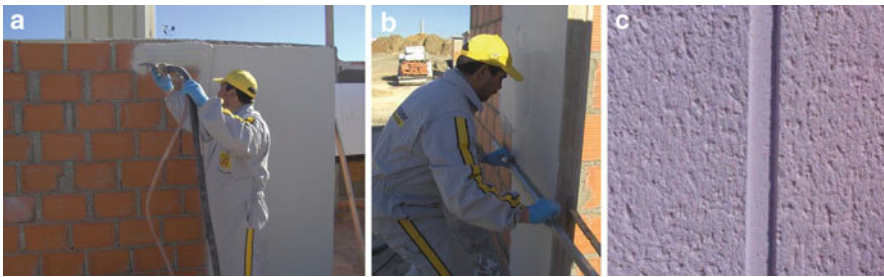
Fig. 2.26 (a) Application of one-coat render by spraying; (b) pressing and levelling with aluminium ruler; (c) final aspect of a mortar joint
