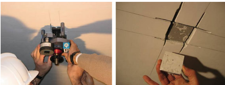
Fig. 3.7 Pull-out test and adhesive failure in the interface between the ceiling's gypsum coating and the concrete substrate
