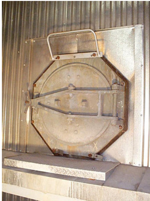
Figure 13.11 Insulation of the furnace wall, also showing a manhole.
