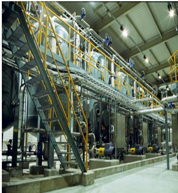
Figure 8.7 Feedwater treatment plant.
