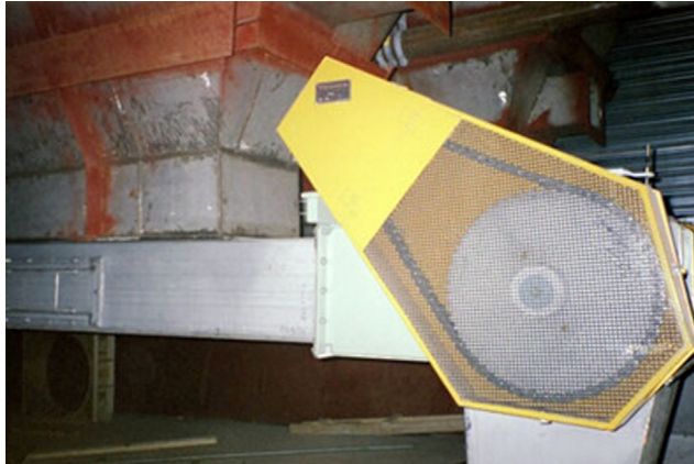
Figure 6.13 Typical ash conveyor before insulation.
