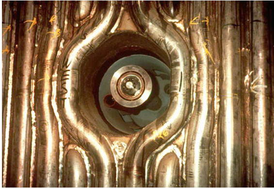
Figure 6.3 Gas burner at the furnace wall.
