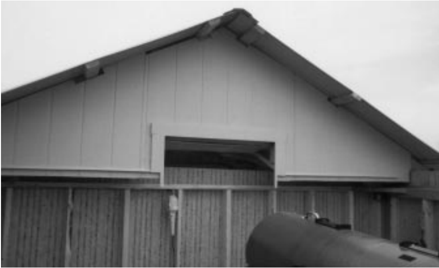
Figure 1.5 1 in \times 6 in trim added to the southern wall and door frame.
