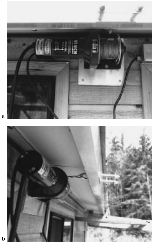
Figure 21.8 a The winch used for raising and lowering the roof. b The U-bolt cable-connection and shock-absorbing springs.
