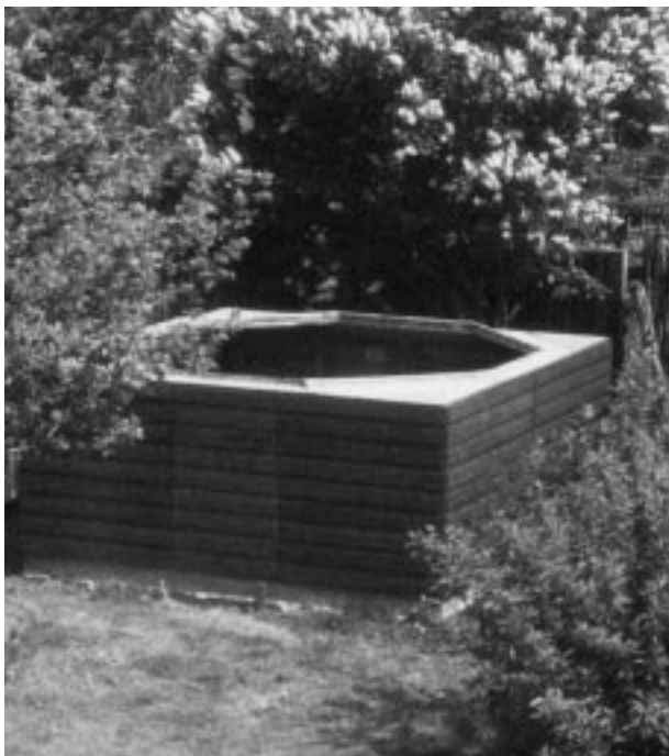
Figure 11.2 The observatory walls completed, together with the flat roof areas and internal timber upstand.
