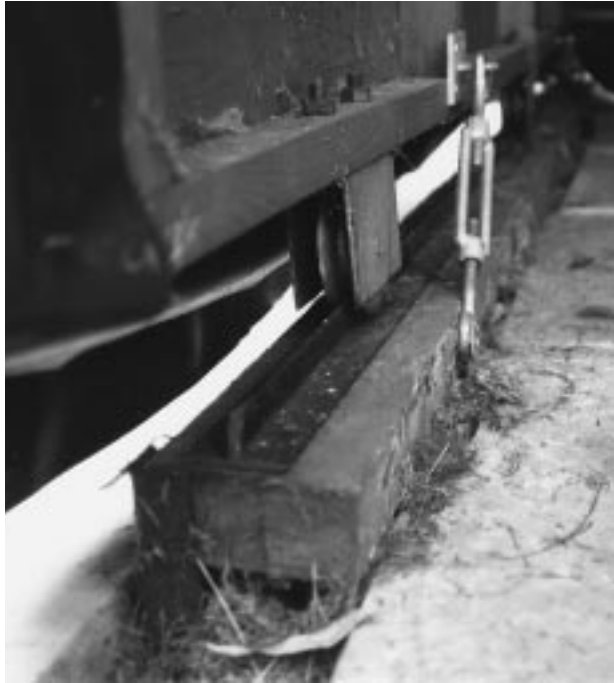
Figure 20.2 Close-up of the inverted “T”-section rail and one of the V-groove pulley blocks. Also note the turnbuckle fastener used to secure the shed to the rail timber.
