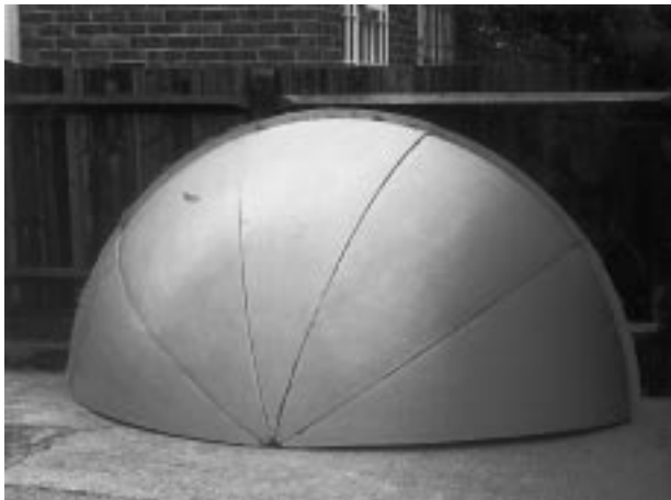
Figure 11.3 The first five dome panels assembled to enable overall dimensions to be checked prior to erecting the panels on the observatory.
