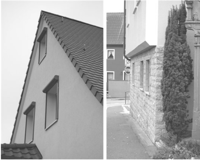
Fig. 2 Left A thick insulation layer influences the façade view at the interface façade/window. Right Not completed insulation due to the fact that the insulation had to be mounted close to the surrounding property
