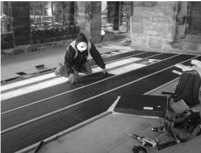
Fig. 16 Preparation of the support structure containing the VIP panels. The used VIPs of type ‘va-Q-vip B’ have an additional protection layer, which is responsible for the blackish colour of the VIPs
