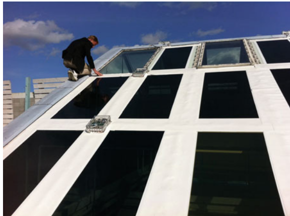
Fig. 17 Test installation of a foil-based electrochromic glazing on a skylight used in a supermarket in Uppsala, Sweden, during 2012–2013. From Gregard (2012)
