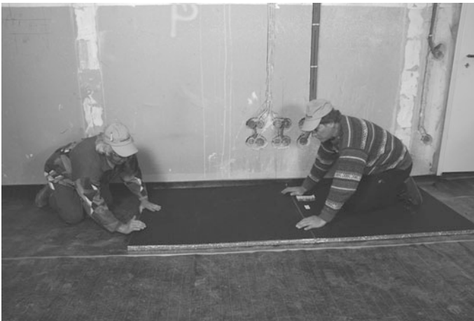
Fig. 21 Installation of the VIP at the floor at the top of a vapour barrier. The VIPs of the type Vacupor RP-B2-S were laminated with a building protective mat
