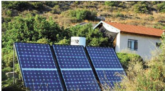
Fig. 16 ‘MULTI SOLAR’ PV/T system from ‘Millennium Electric’ (Zhang et al. 2012)
