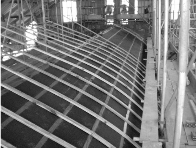
Fig. 17 Mounted VIP construction with wooden framework for the final metal roof sheets
