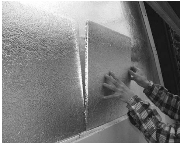
Fig. 11 Installation of the VIP on the top of the vapour barrier. In the edge regions, triangular-shaped VIPs were used
