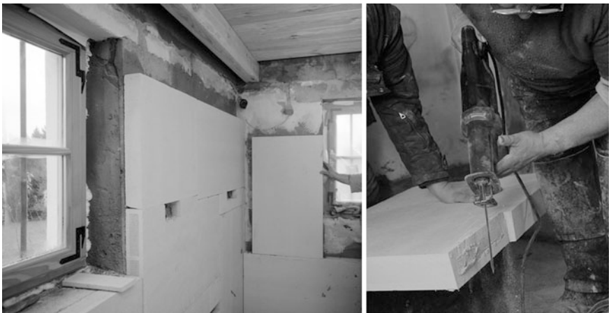
Fig. 28 Installation of the interior thermal insulation with CALOSTAT ® in combination with a calcium silicate insulation material ( left picture ). Right picture The calcium silicate board with microporous insulation kernel, i.e. CALOSTAT ® , allows a time and cost-efficient installation and an individual adjustment at the construction site
