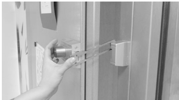
Fig. 13 Sonderschule 4: catches to keep door open allowing night cooling. Photo Xavier Dequaire
