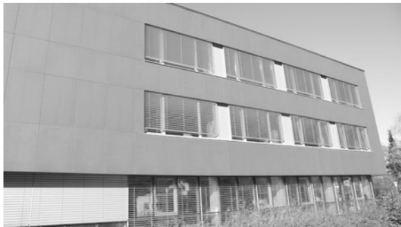
Fig. 10 Zams-Schönwies, south façade after upgrade: columns are inside the new thermal envelope. Photo Xavier Dequaire
