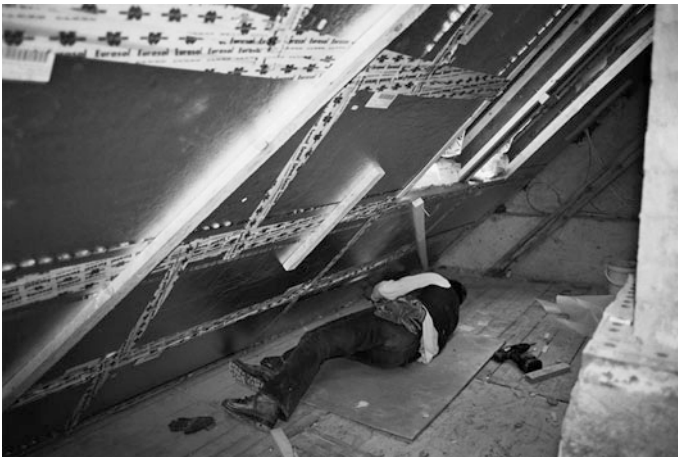
Fig. 19 Same attic as in Fig. 18. Also, the vertical discontinuities are sealed and a wooden framework is mounted for the installation of gypsum plaster boards
