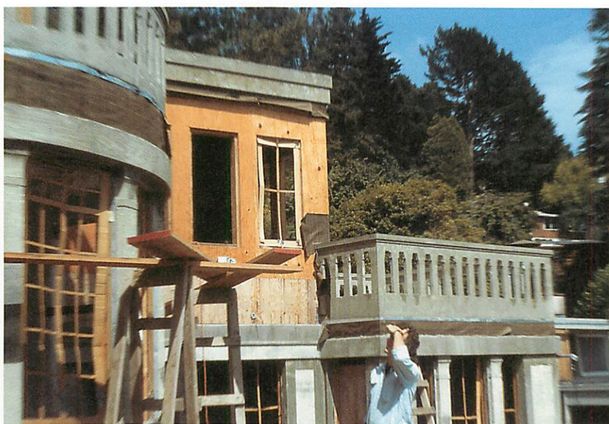
Before ordering windows, we made cardboard mockups of the glazing bar and pane layout in every window in the house, and examined them from inside for their effect on the room, and from outside for their effect on the street
