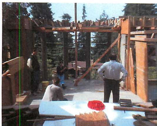
Upham house: settling positions of columns, to form the bays, and window openings of the living room bay window.
