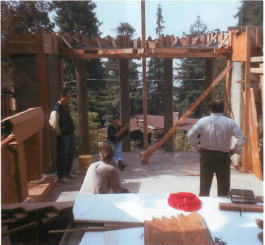
Settling positions of columns, to form the bays and window openings of the living room bay window
