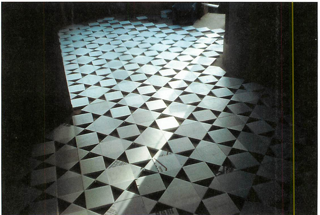
Styrofoam forms from the making of the kitchen floor, in preparation for the first colored terrazzo to be poured into the voids between the pieces of styrofoam (white)
