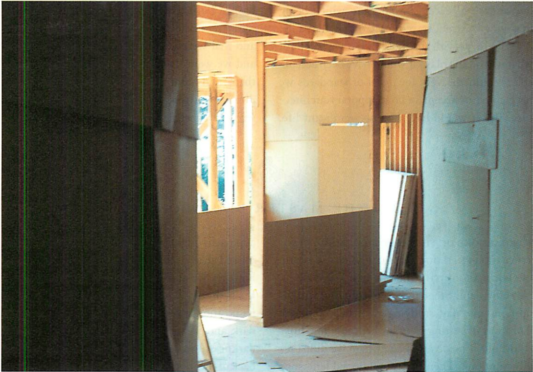
The upstairs after rough framing, and before new decisions were made. The cardboard walls and mocked-up partitions showed us clearly just how bad it was.
