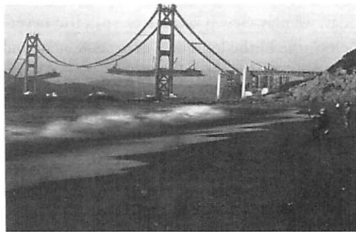
The cables, completed, hang loosely across the towers, before the vertical cables are put in place.
