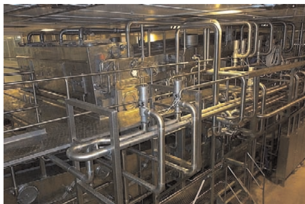
Figure 6 APV Cheddarmaster belt system. Courtesy of Fonterra Cooperative Group, New Zealand.
