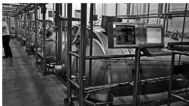
Figure 1 Large-scale manufacture of LMPS Mozzarella cheese in a series of enclosed cheese vats.
