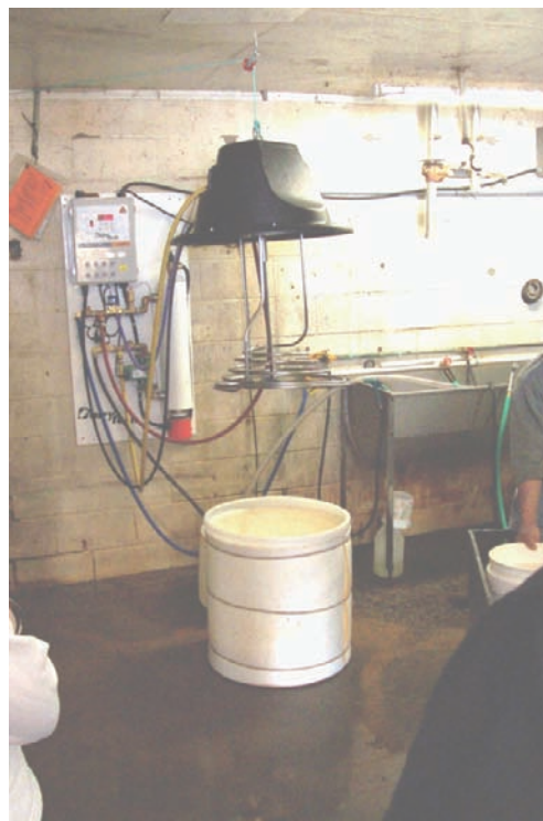
Figure 1 Example of a batch pasteurizer system (Dairy Tech, Windsor, CO).
