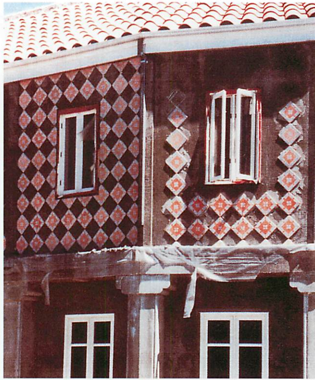
Two versions of the way the tile repeat might meet the window, before the final tile work was set. Though unusually hard to decide, it slowly became clear that the right-hand version created an atmosphere of greater wholeness in an observer, and that was the one we chose. The extra gray space around the window, though at first sight less complete and less perfectly made, induced a greater feeling of relatedness than the left-hand example which was more conventional, and more "perfect."
