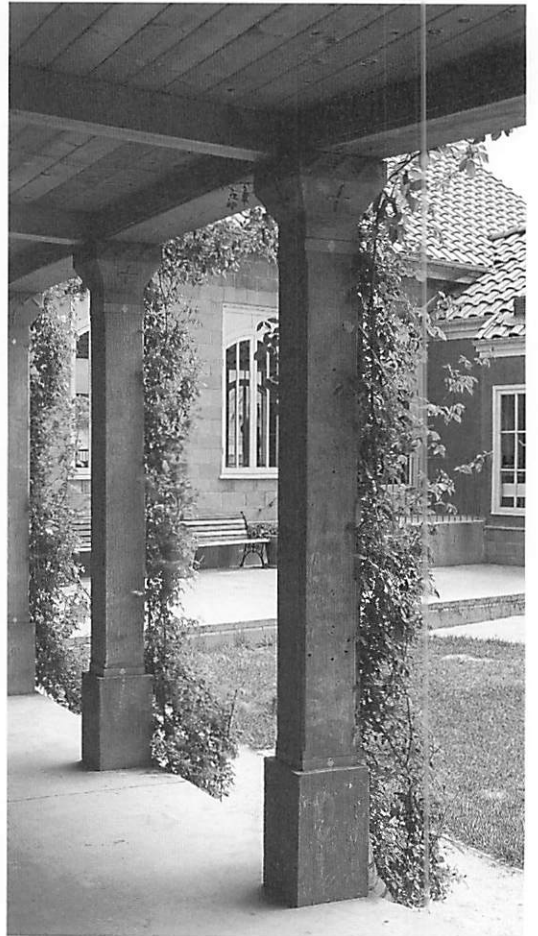
The experimental columns, installed in a colonnade in the Julian Street Inn, San Jose, California.
