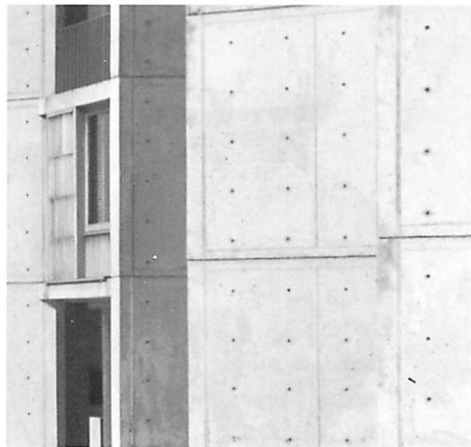
Concrete wall. A jump in scale of 2000 to 1 from panel to bolt-heads, too huge to create levels of scale effectively at all.
