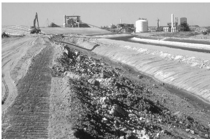
Fig. 7.5 Phosphogypsum stack at the Phosphate Hill mine, Australia. The dry phosphogypsum is reslurried prior to disposal and discharged onto the top of the stack where the solids settle. Waters (pH 1.5) seep through the stack and are collected in circumscribing plastic lined ditches
