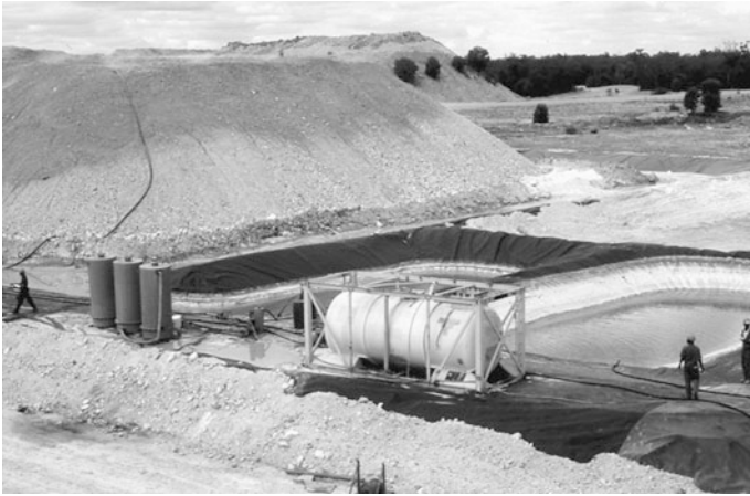
Fig. 5.4 Cyanide heap leach pile and plastic lined collection ponds, Wirrallee gold mine, Australia
