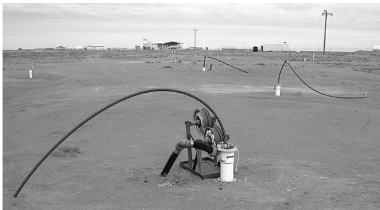
Fig. 6.4 Borefield of the Honeymoon ISL uranium mine, Australia. An acid leach process is applied to a confined aquifer
